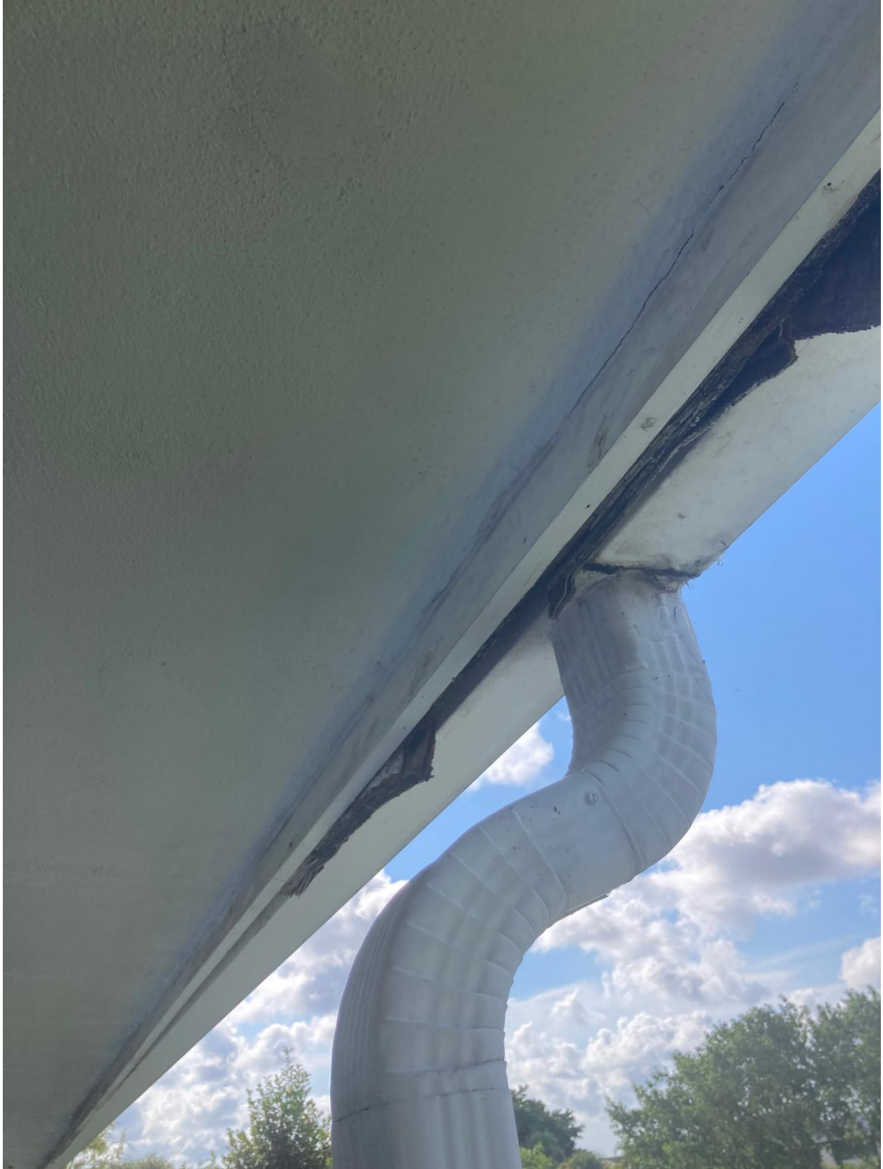
SOMERSET J- ROOF EAVES ARE ROTTED.
