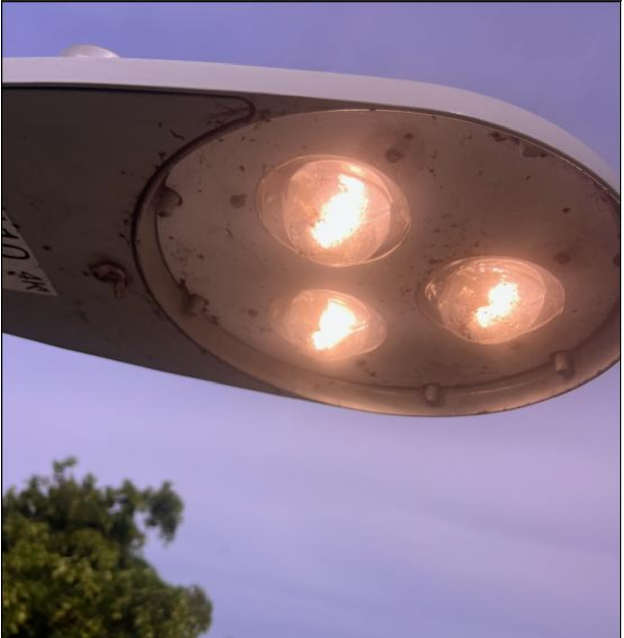
SOUTH DRIVE- THIS STREETLIGHT NEAR WELLINGTON J WAS REPAIRED BY FPL ELECTRICIANS ON 8/5.
