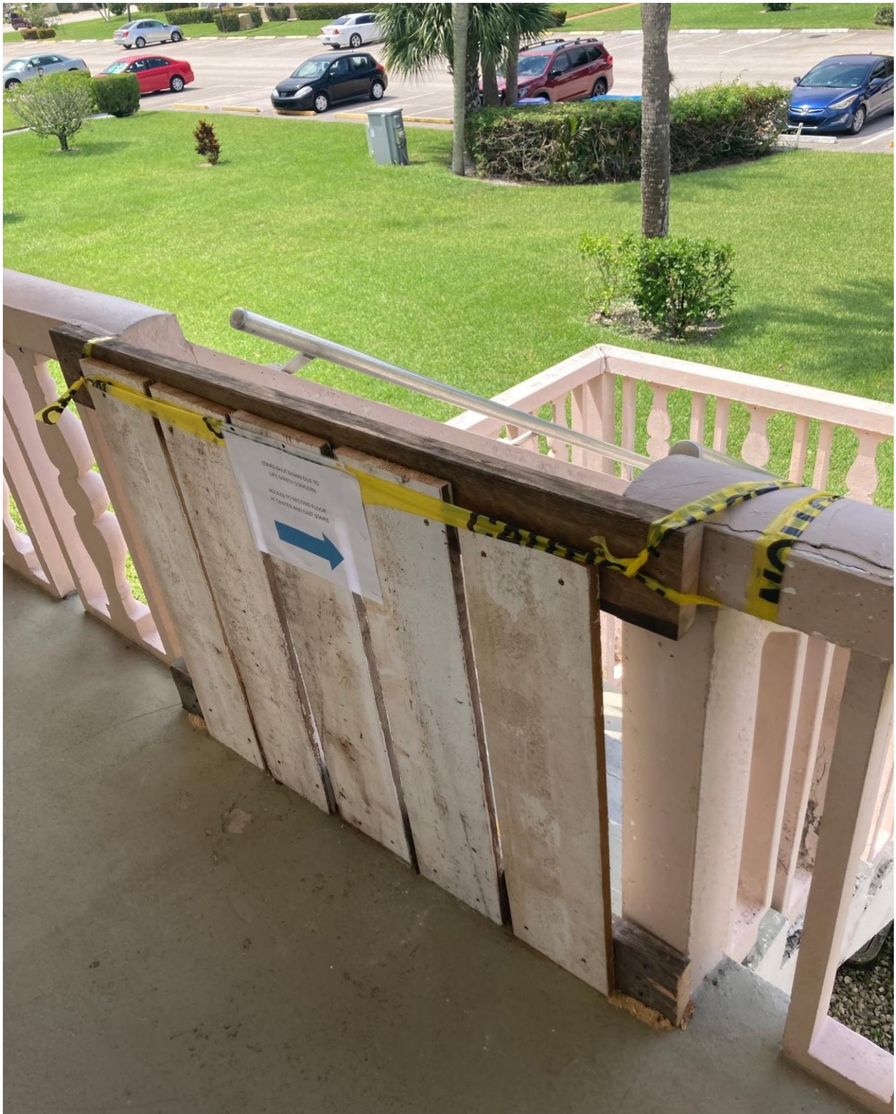
NORWICH B- SEACREST SERVICES BLOCKED OFF THIS UNSAFE STAIRCASE, PER THE SPECIAL MAGISTRATE'S INSTRUCTIONS.
