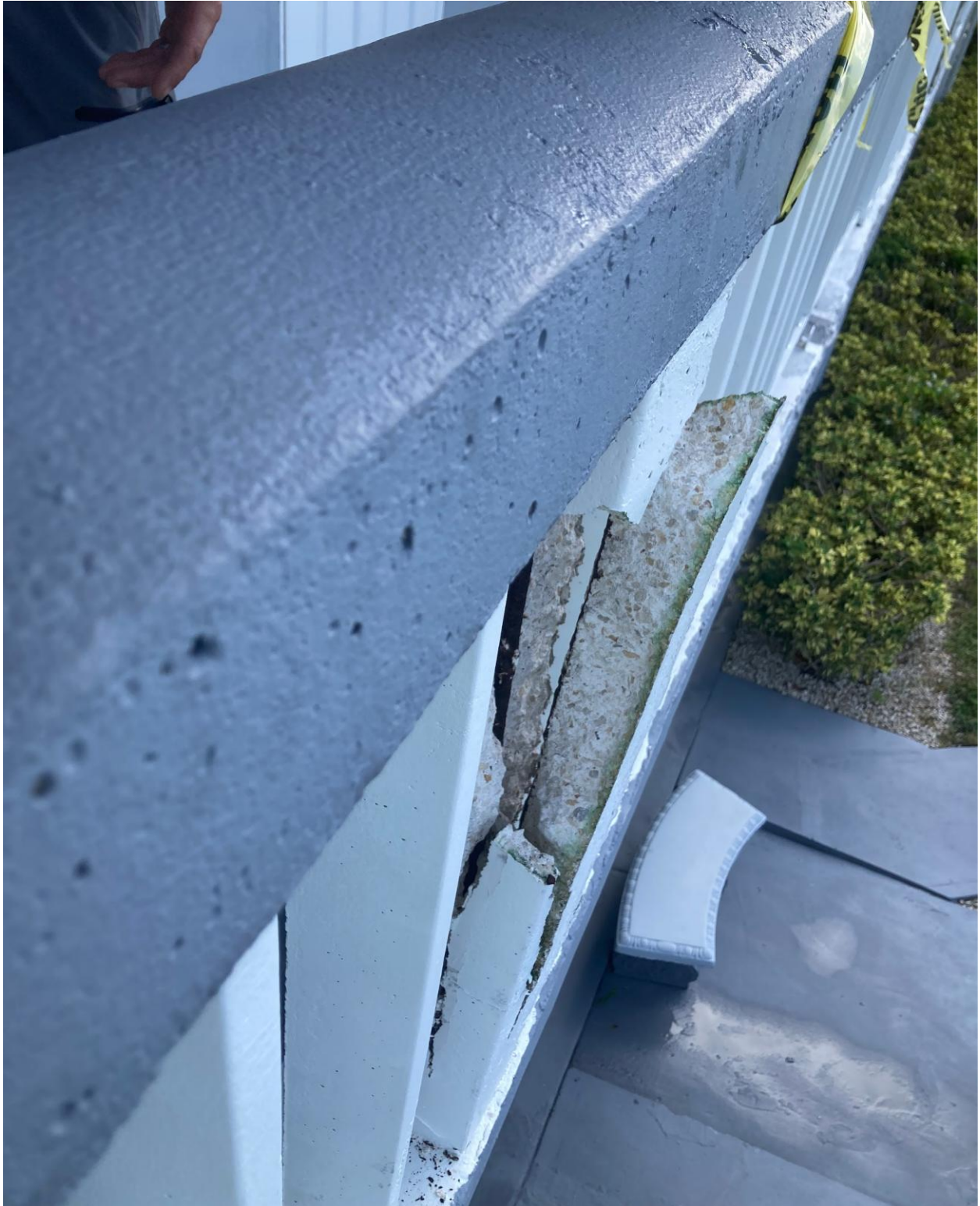
SOMERSET J- THIS RAILING IS SEVERELY DETERIORATED, A LIFE SAFETY RISK.
