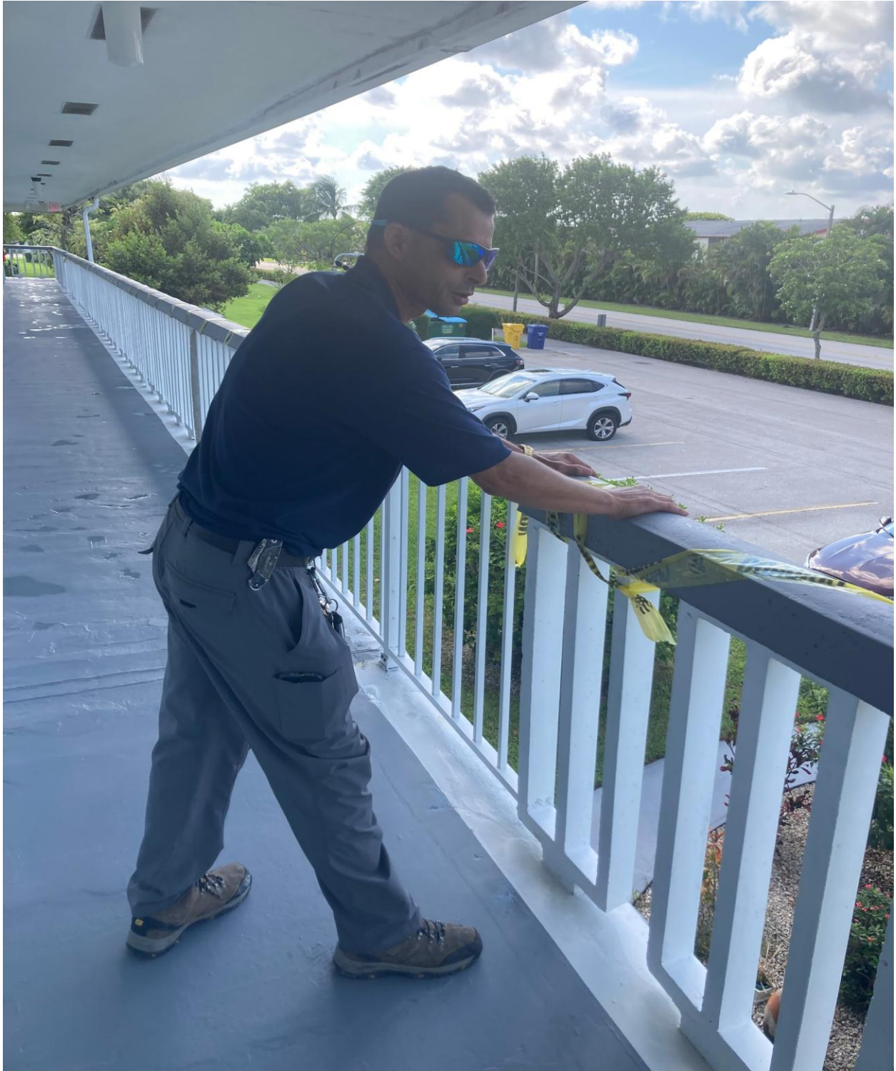
SOMERSET J- SEACREST JOE MENCHI WAS ABLE TO ROCK THIS DETERIORATED RAILING- ONE SOFT HIP BUMP WOULD SEND A PERSON OVER THE SIDE. NOT GOOD.
