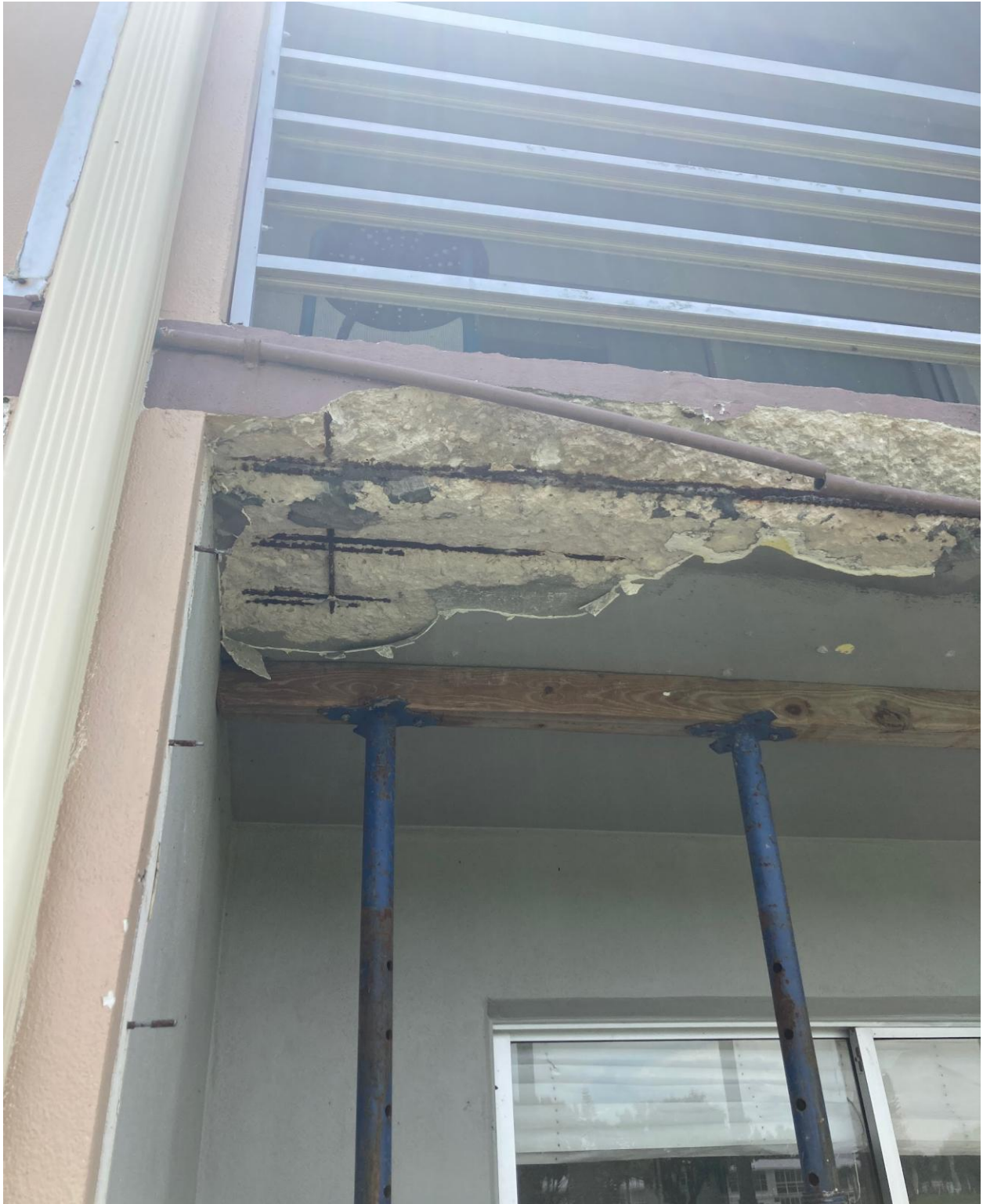
204 SOMERSET K- THIS CONCRETE SLAB, WHICH IS A STRUCTURAL ELEMENT OF THE BUILDING, WAS DAMAGED BY THE UNIT OWNER'S CONTRACTOR.
