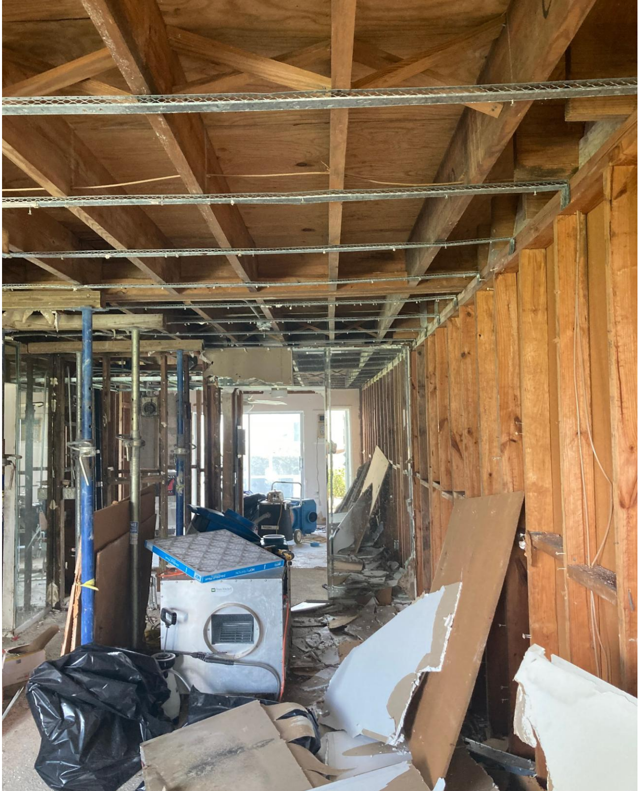
172 COVENTRY H- THIS LOWER UNIT IS NEAR COMPLETELY GUTTED. ALL MOLD CONTAMINATED DRYWALL HAS BEEN REMOVED BY DEAN MITCHELL RESTORATION.
