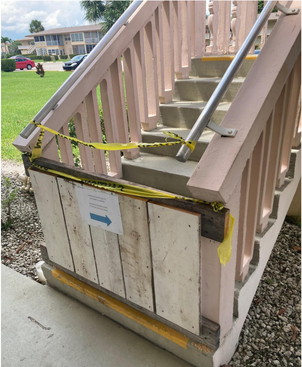
NORWICH B- SEACREST SERVICES BLOCKED OFF THIS UNSAFE STAIRCASE, PER THE SPECIAL MAGISTRATE'S INSTRUCTIONS.
