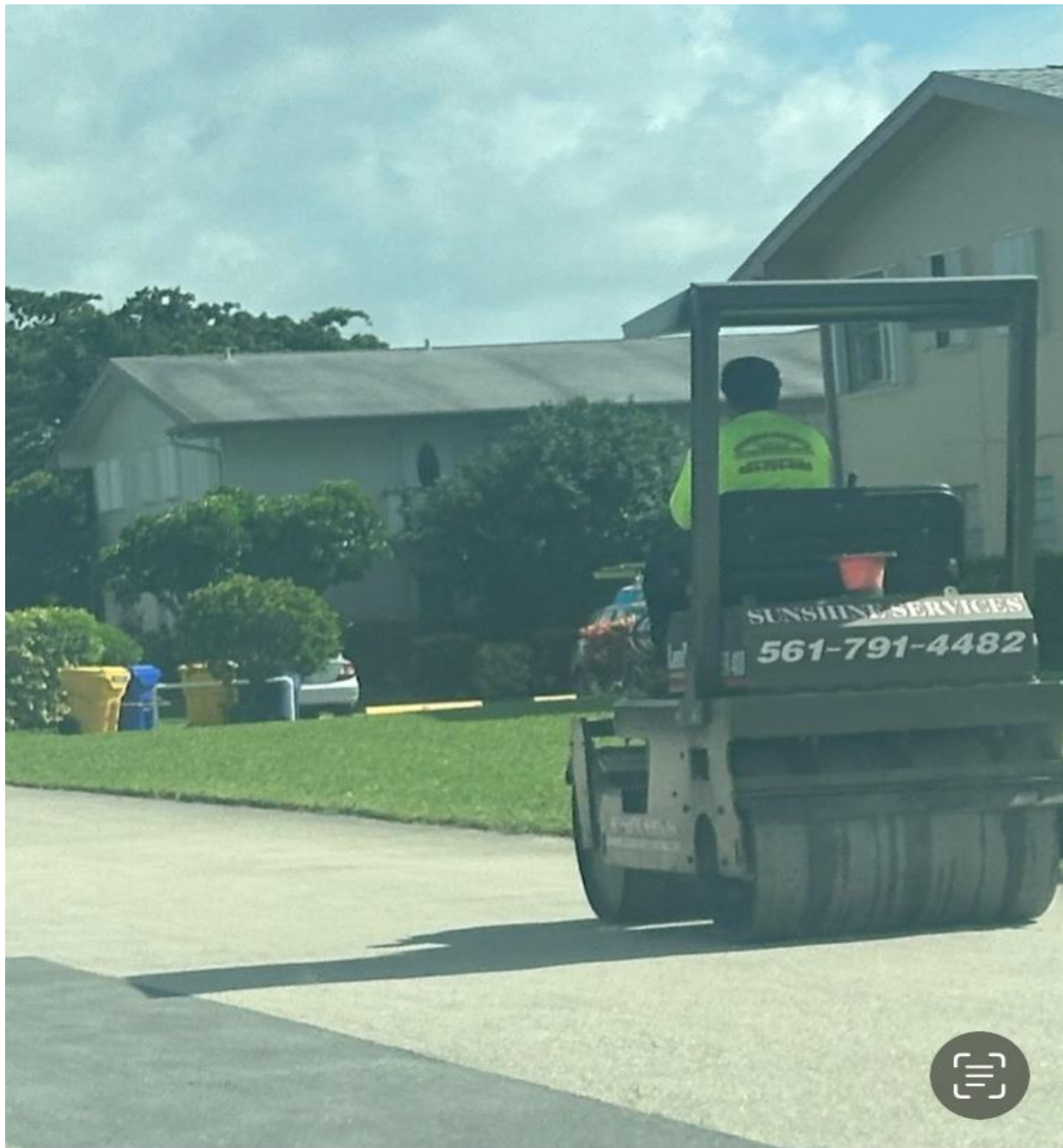
ON 7/3, SUNSHINE SERVICES MADE REPAIRS TO ROADS AND WALKWAYS AT VARIOUS SECTIONS OF CV.
