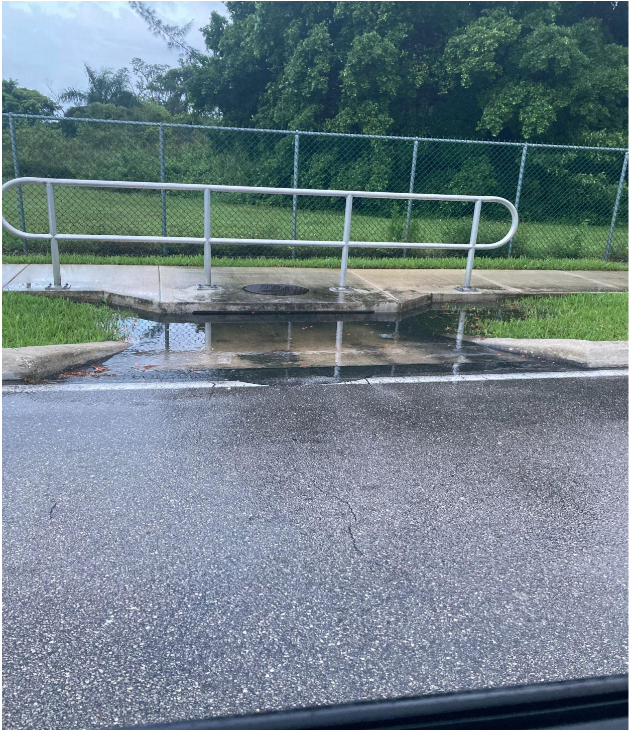
CENTURY BOULEVARD- ON 7/1, ANCHOR MARINE CLEARED STORMWATER CATCH BASINS ALONG THE SOUTH SIDE OF CENTURY BOULEVARD. THIS ONE WAS COMPLETELY BLOCKED.
