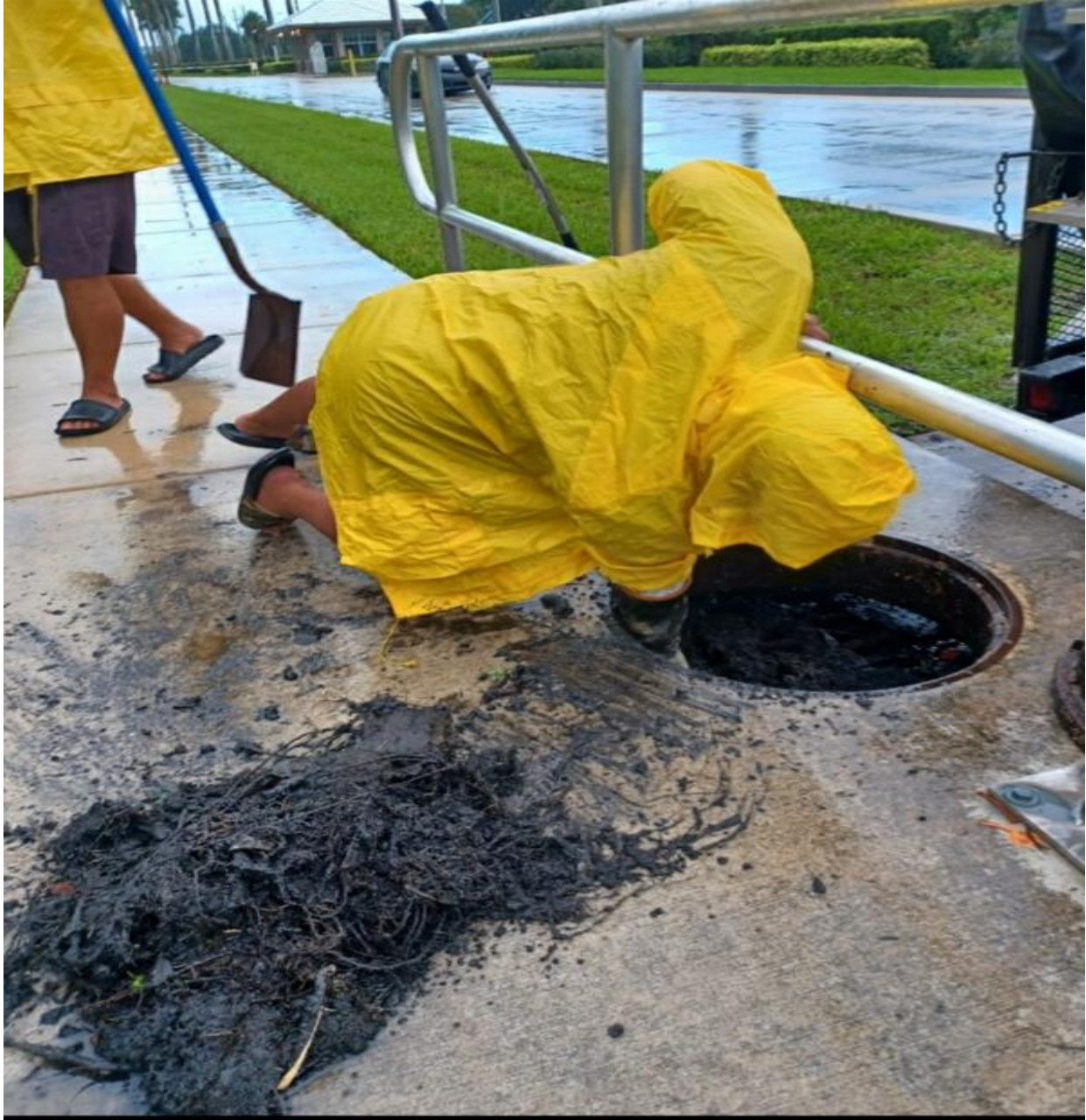
CENTURY BOULEVARD- ON 7/1, ANCHOR MARINE CLEARED STORMWATER CATCH BASINS ALONG THE SOUTH SIDE OF CENTURY BOULEVARD.
