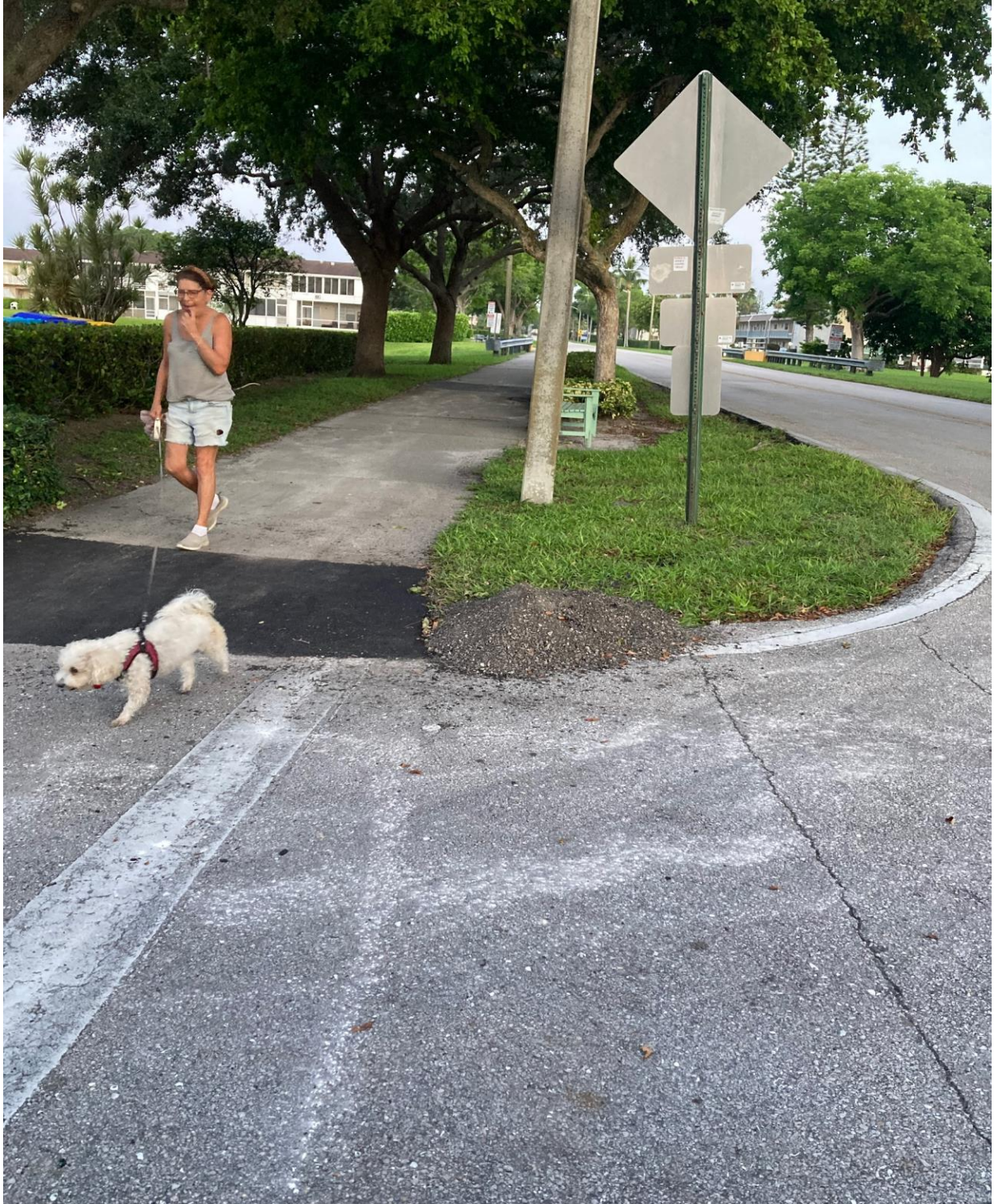
STRATFORD SECTION- WALKWAY REPAIR COMPLETE. I CALLED THE VENDOR TO RETURN AND REMOVE THAT PILE OF FILL NEXT TO THE REPAIR AREA.
