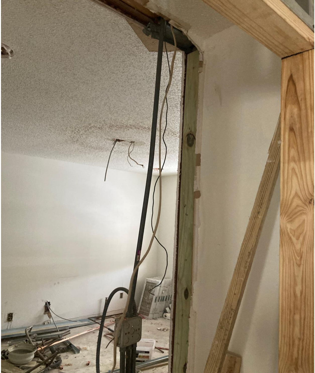
165 STRATFORD L- MAJOR ELECTRICAL WORK HAPPENING HERE, WITH NO ELECTRICAL SUB PERMIT AND NO ENGINEERING PLANS.
