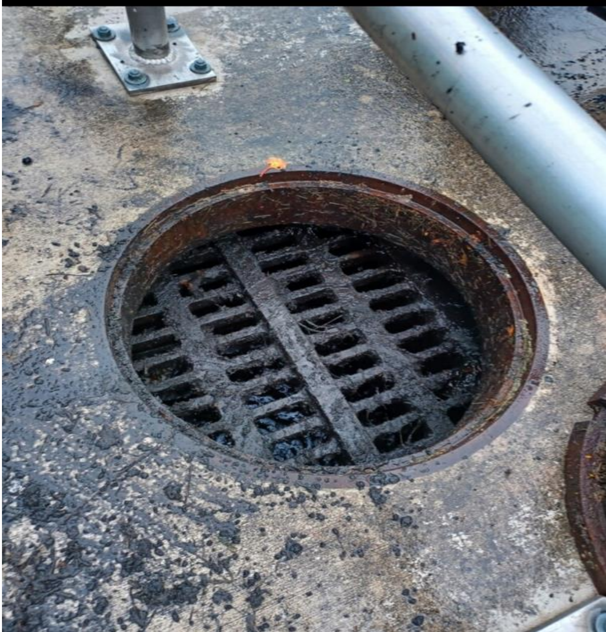
CENTURY BOULEVARD- STORMWATER CATCH BASINS ON THE SOUTH SIDE OF CENTURY BOULEVARD ARE CLEAR.
