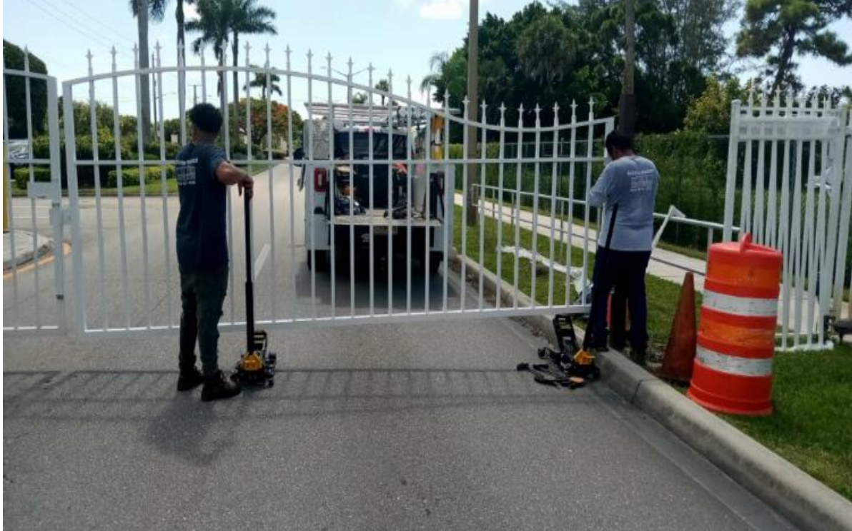
CENTURY BOULEVARD- NEW SWING GATE INSTALLED BY ACCESS MASTERS ON 7/26, REPLACING ONE THAT WAS PREVIOUSLY SMASHED BY A TRUCK.
