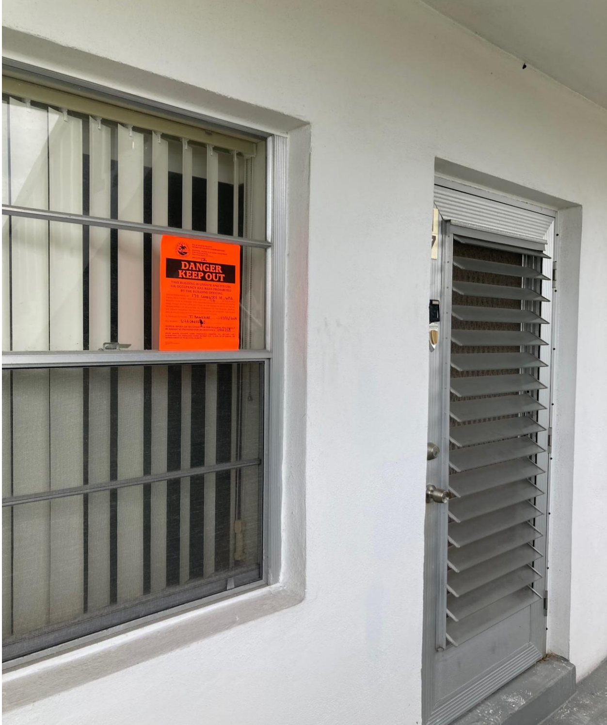
172 COVENTRY H- THIS UNIT HAS BEEN “RED-TAGGED” BY PZB BUILDINGS DEPARTMENT AS UNSAFE FOR OCCUPANCY. POST SHORING WILL NEED TO BE INSTALLED TO MAKE THESE UNITS SAFE FOR THE WORKERS.
