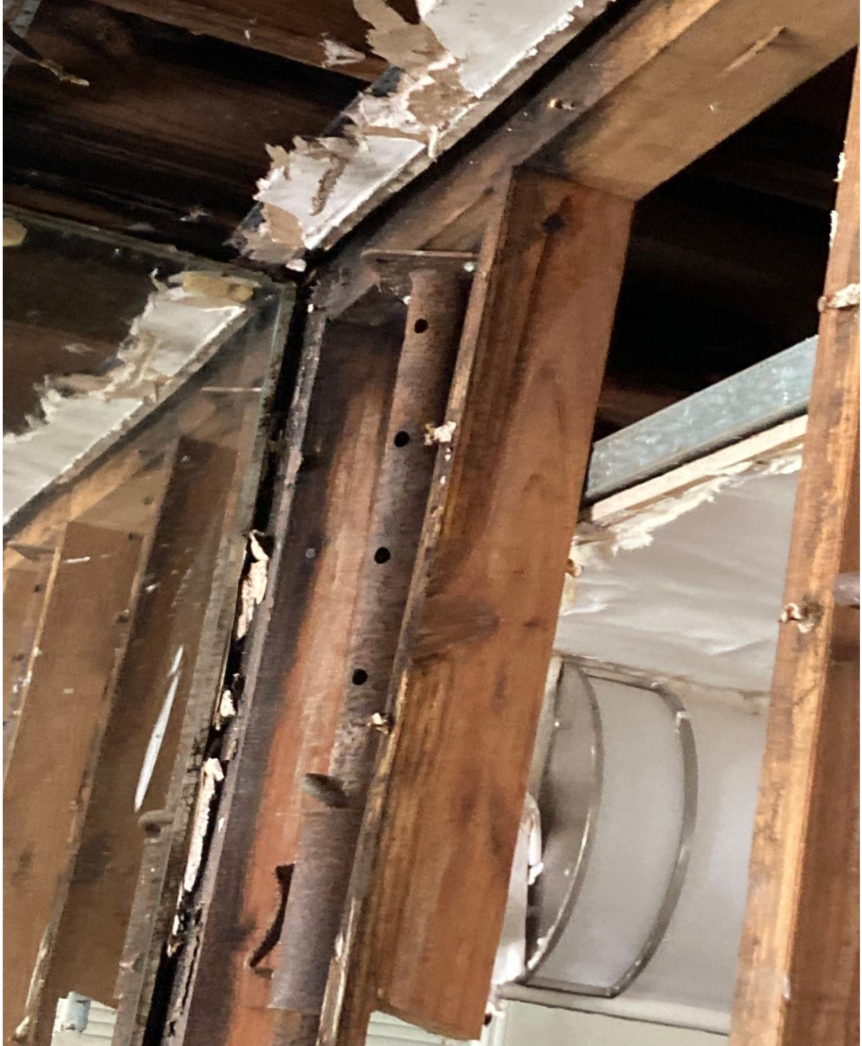
170 COVENTRY H- THIS WOOD GIRDER IS SEVERELY COMPROMISED, AND EXTENDS INTO AN ADJACENT UNIT.
