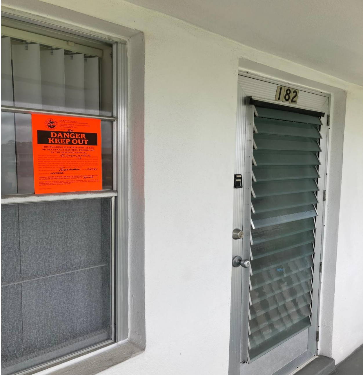
182 COVENTRY H- THIS UPPER UNIT, THE SOURCE OF THE LEAK, WAS “RED-TAGGED” BY PZB BUILDING INSPECTORS ON 7/23. THIS UNIT IS UNSAFE FOR OCCUPANCY. THE INSPECTORS SUSPECT THAT THE WOOD FLOOR HAS BEEN COMPROMISED BY WATER DAMAGE. AN STRUCTURAL ENGINEER WILL NEED TO INSPECT THIS BUILDING.
