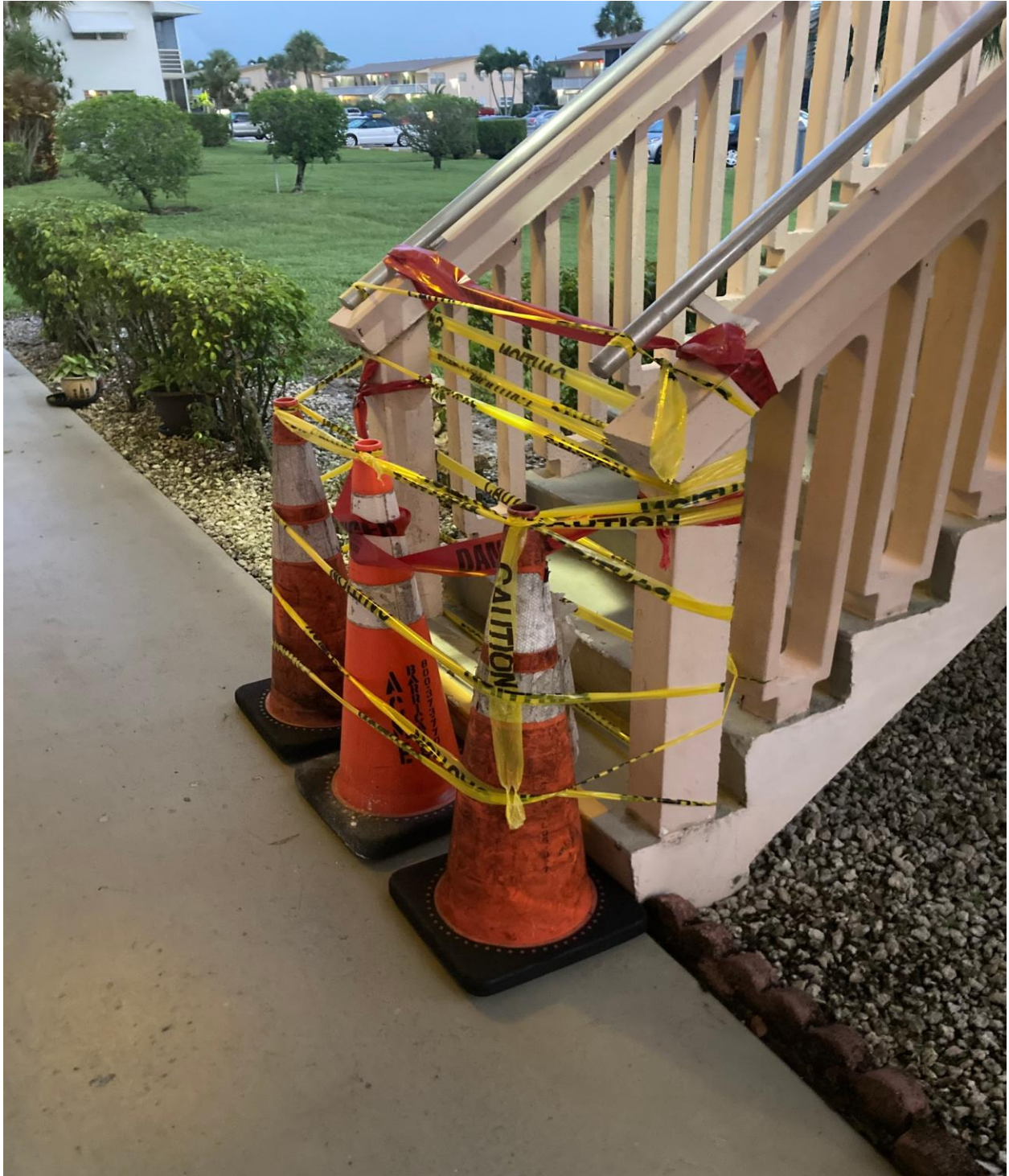
NORWICH B- ON 7/22, PLATINUM SECURITY BARRICADED THIS UNSAFE STAIRWAY AT TOP AND BOTTOM.
