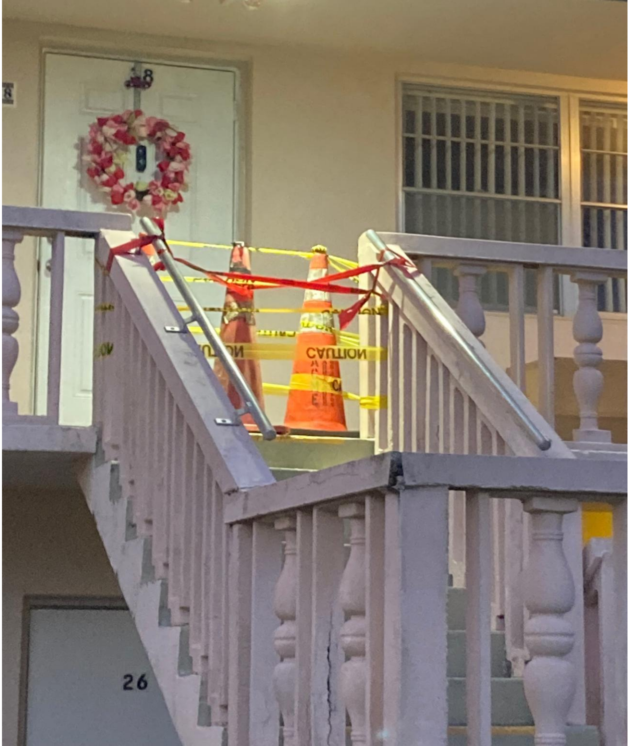
NORWICH B- THIS STAIRCASE IS UNSAFE FOR USE.
