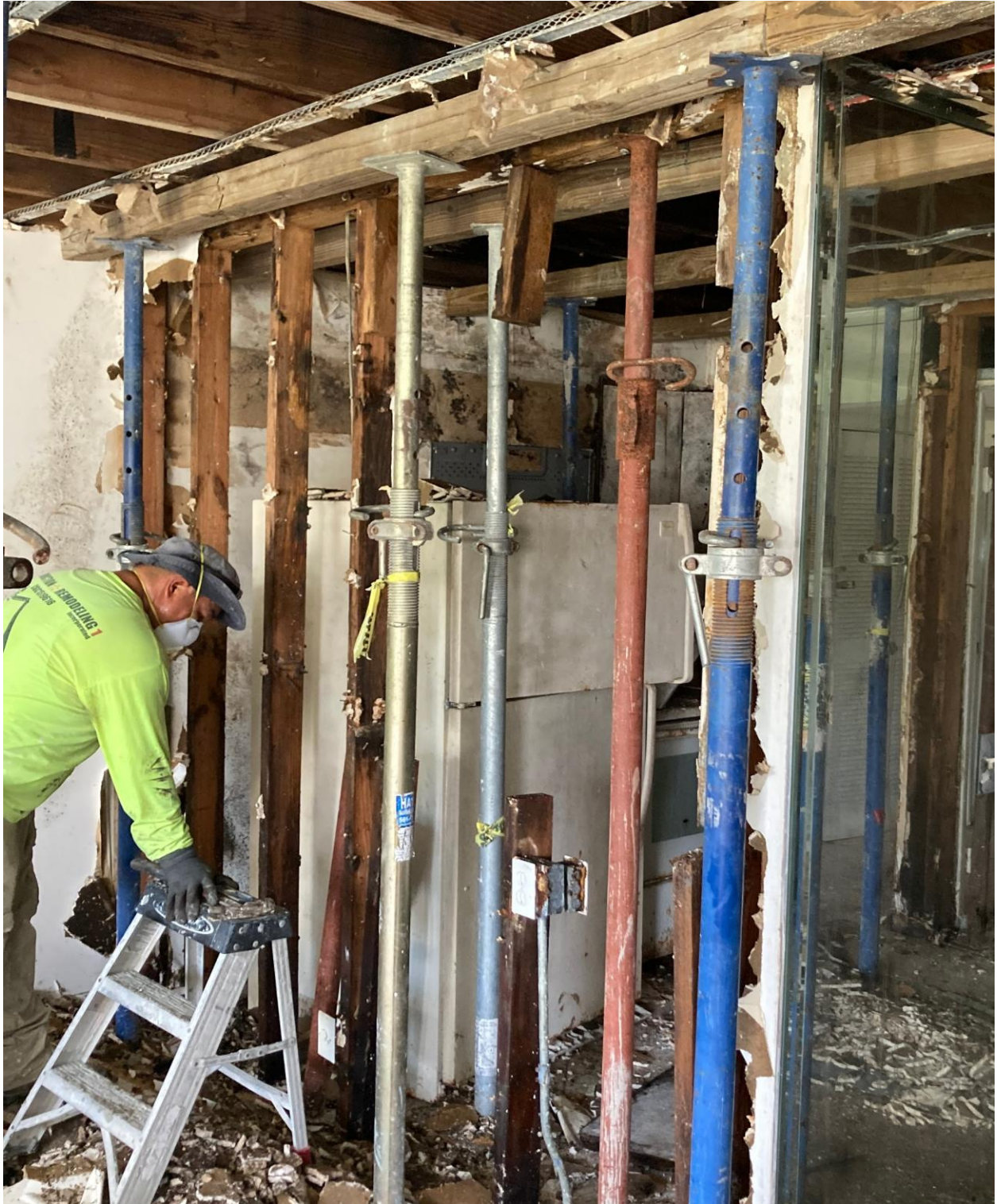
170 COVENTRY H- THIS LOAD BEARING KITCHEN WALL IS ALSO ROTTED.
