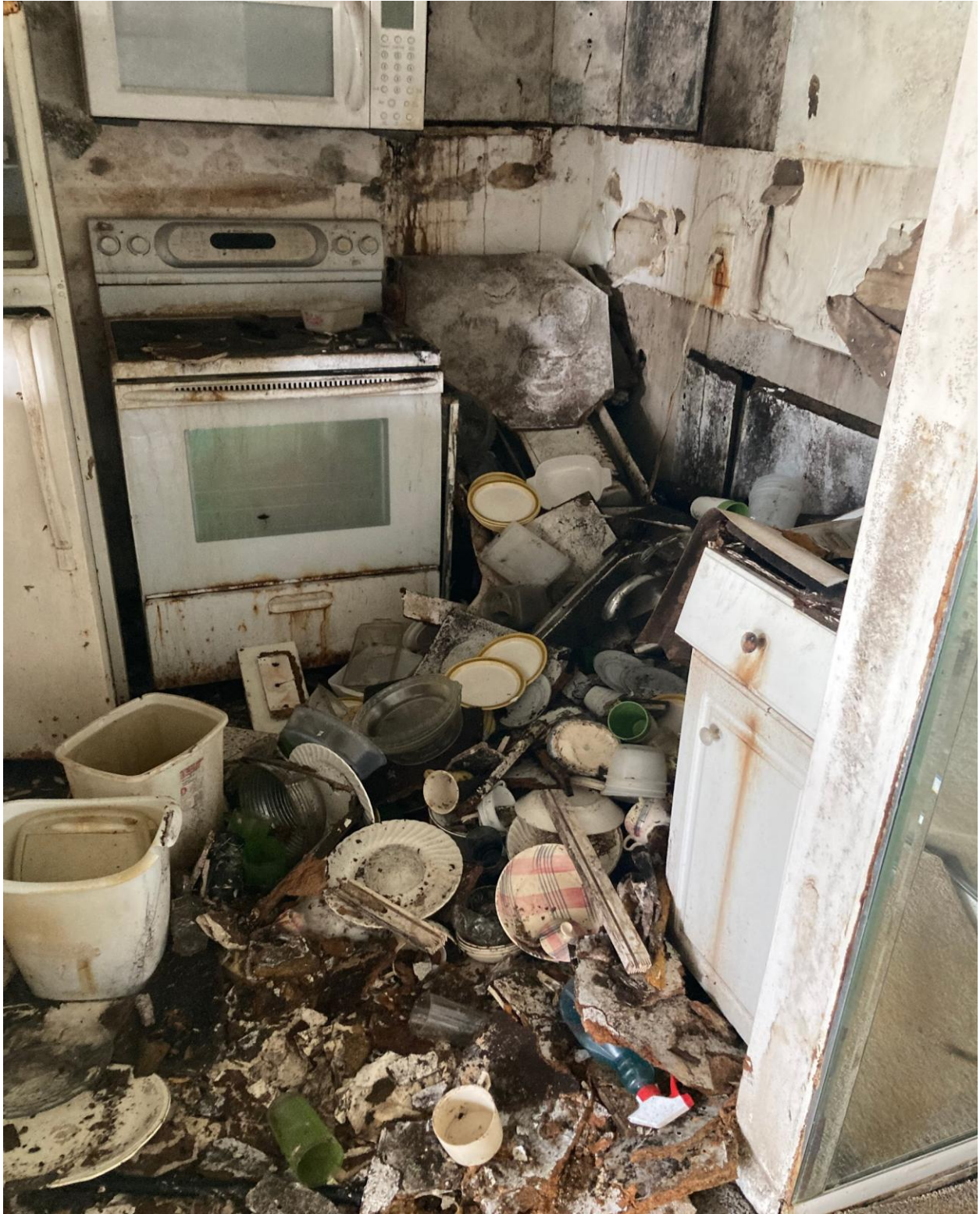
170 COVENTRY H- THIS DISASTER WAS REPORTED TO PZB BUILDINGS DEPARTMENT, CASE #C-2024-07220003.
