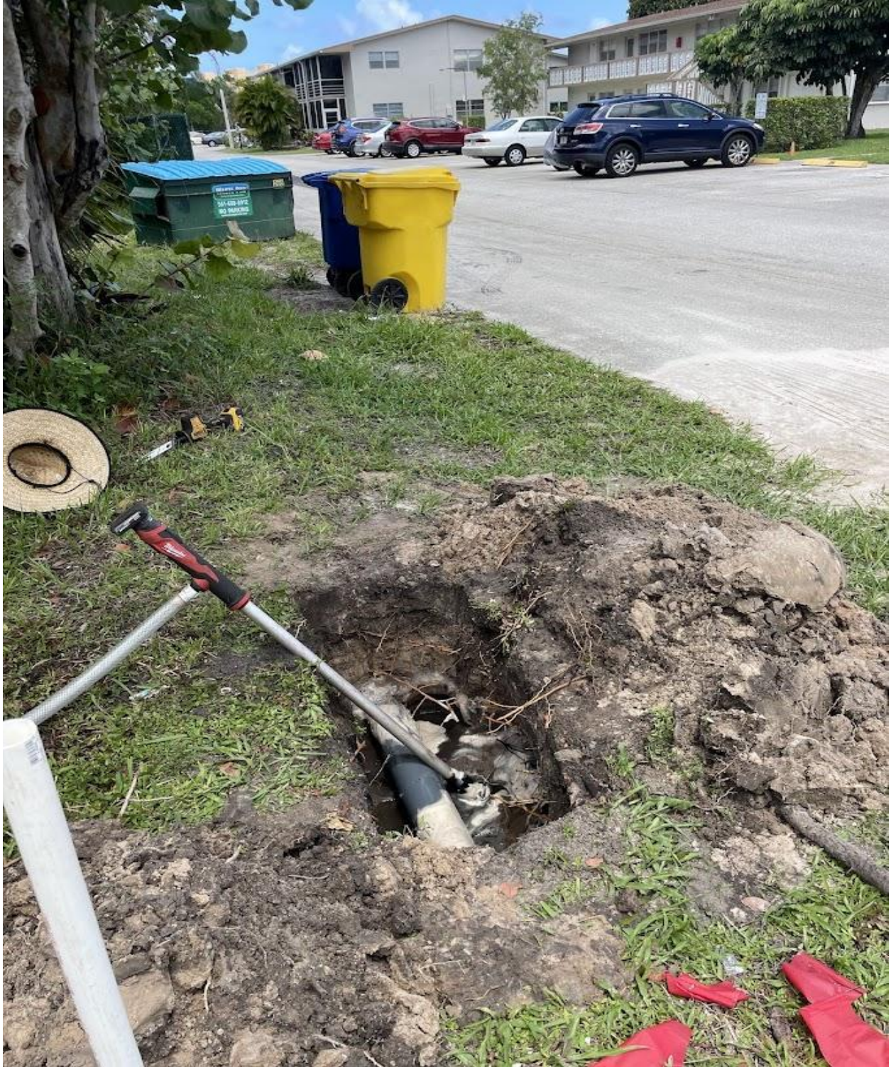
NORWICH SECTION- UNDERGROUND FOUR INCH IRRIGATION PIPE REPAIRED BY SEACREST SERVICES ON 6/21.
