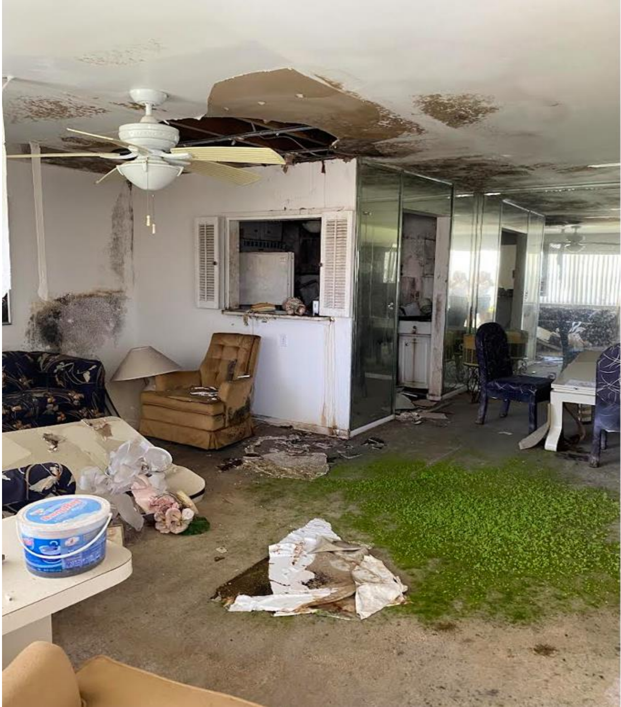
170 COVENTRY H- A LONG RUNNING LEAK CAUSED CATASTROPHIC DAMAGE TO TWO UNITS. GRASS IS GROWING OUT OF THE CARPET.
