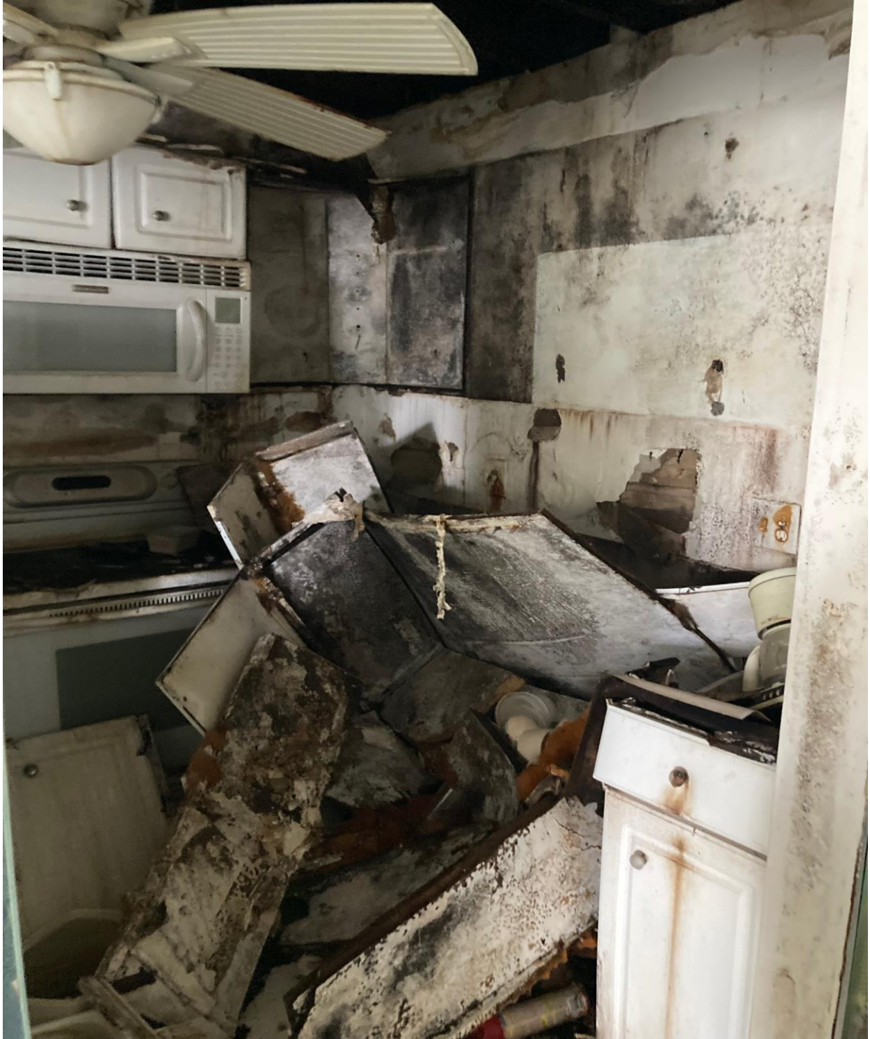
170 COVENTRY H- THIS UNIT, AND THE ONE ABOVE, IS UNINHABITABLE.
