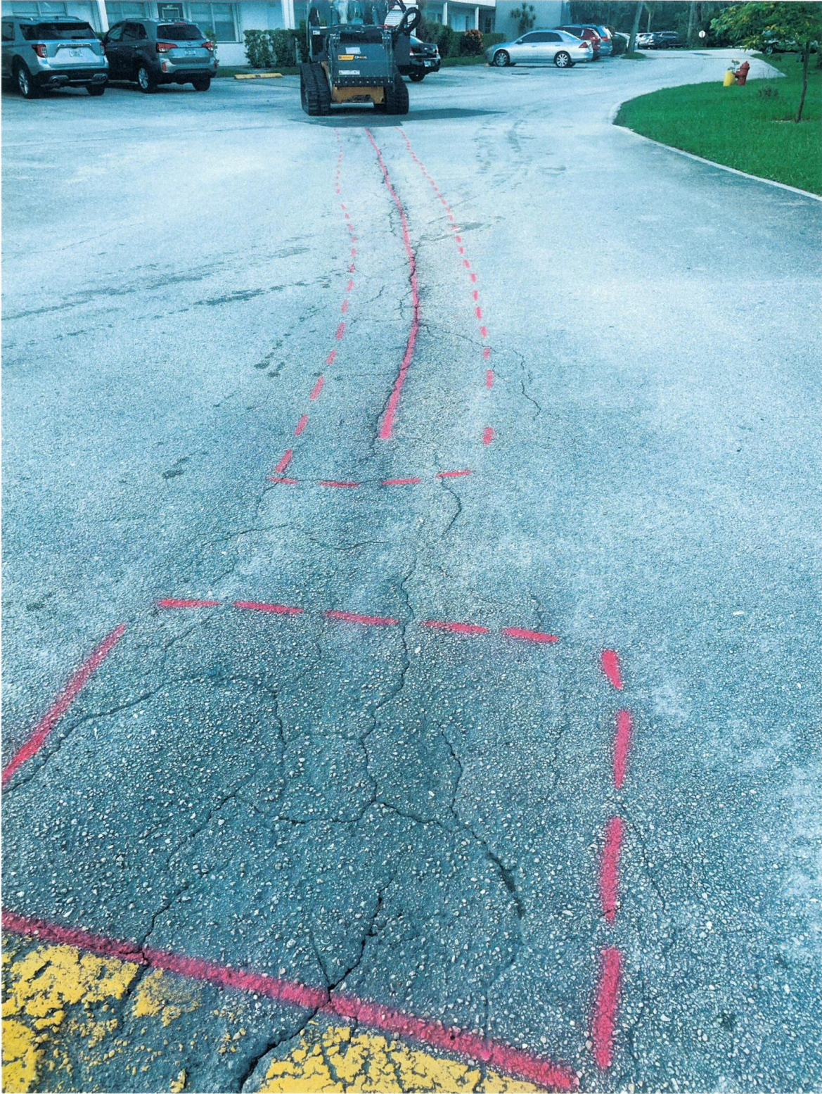
WELLINGTON SECTION- A DETERIORATED SECTION OF ROAD IS MARKED FOR REPAIR.
