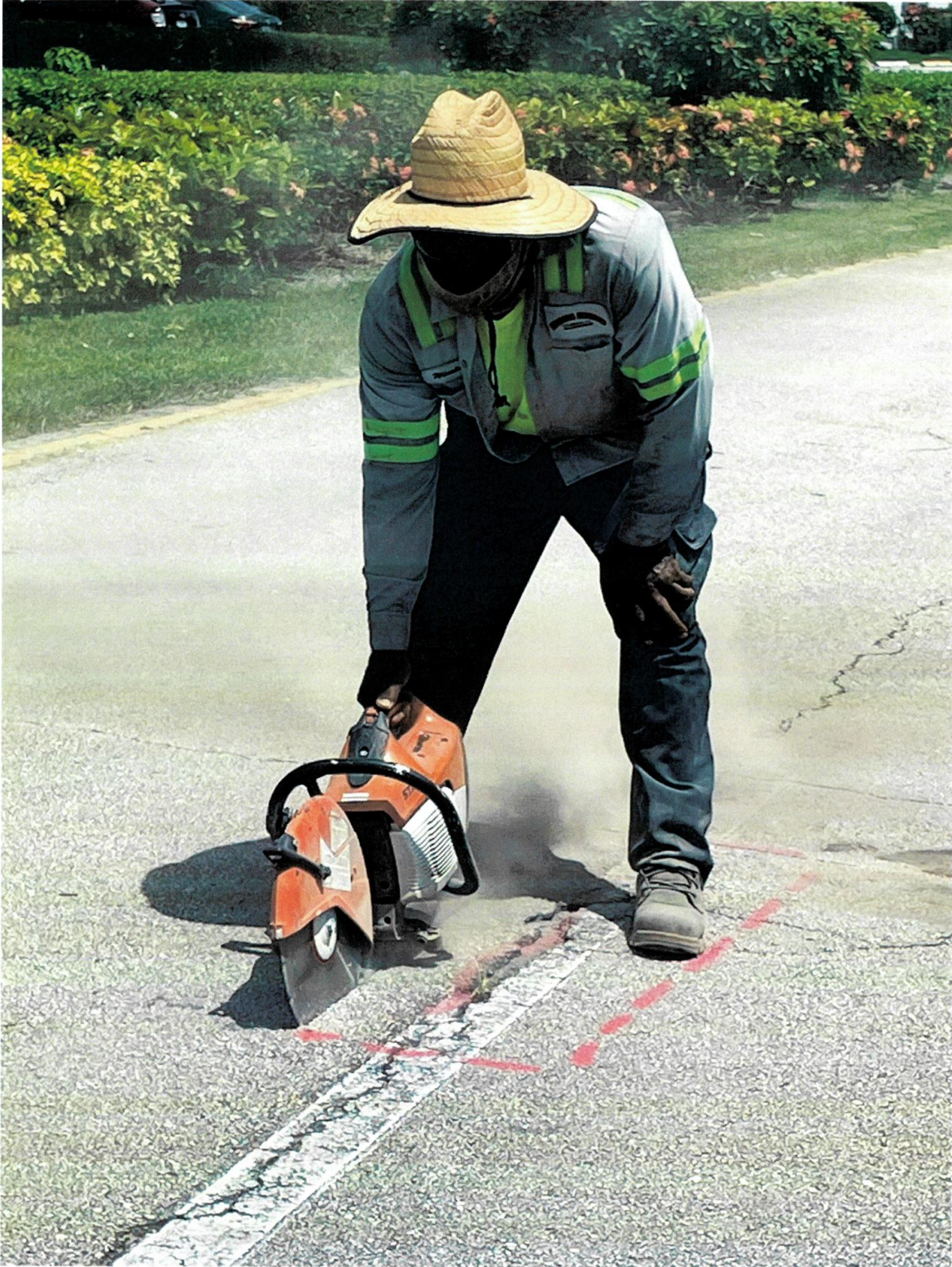
WEST DRIVE- DETERIORATED SECTIONS ARE CUT OUT AND REMOVED FOR A FULL DEPTH REPAIR.
