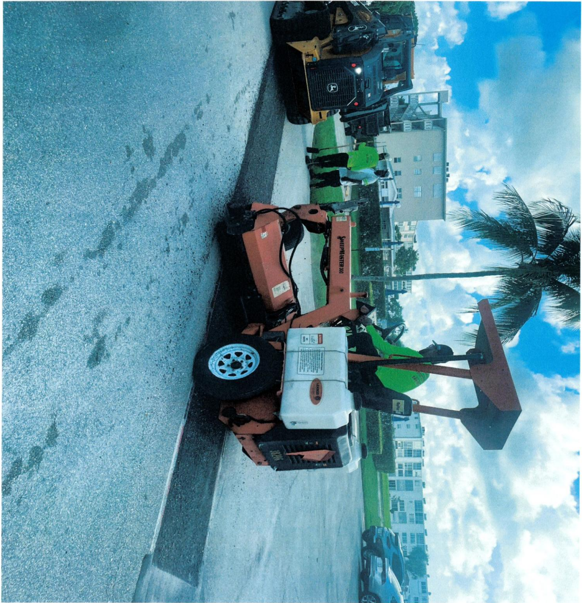
WELLINGTON SECTION- REPAIR AREA IS BRUSHED AND ROLLED, FOR A SEAMLESS PATCH.
