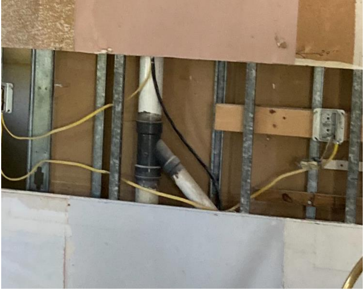
196 WALTHAM H- YIKES! CUT PIECES OF EXTENSION CORDS USED AS ELECTRICAL WIRING. A FIRE WAITING TO HAPPEN.
