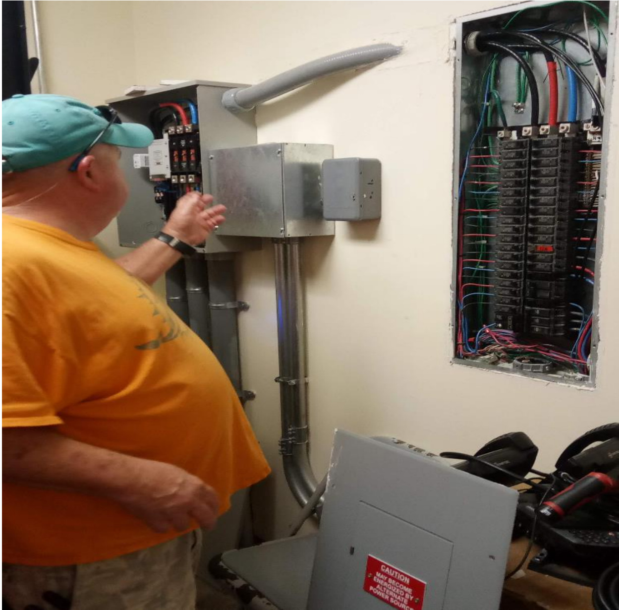
UCO OFFICE- WHILE THE EMERGENCY GENERATOR WAS POWERING THE BUILDING, STEVE CHECKED THE ELECTRICAL PANELS AND AUTOMATIC TRANSFER SWITCH FOR PROPER FUNCTION. ALL GOOD.
