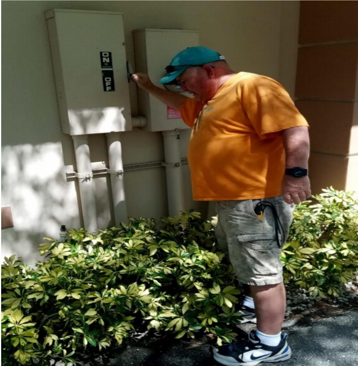
UCO OFFICE- ON 6/21, ELECTRICIAN STEVE BURRIS SHUT DOWN MAINS POWER FOR THE BUILDING. OUR EMERGENCY GENERATOR FIRED RIGHT UP AND POWERED THE BUILDING FOR FIFTEEN MINUTES.
