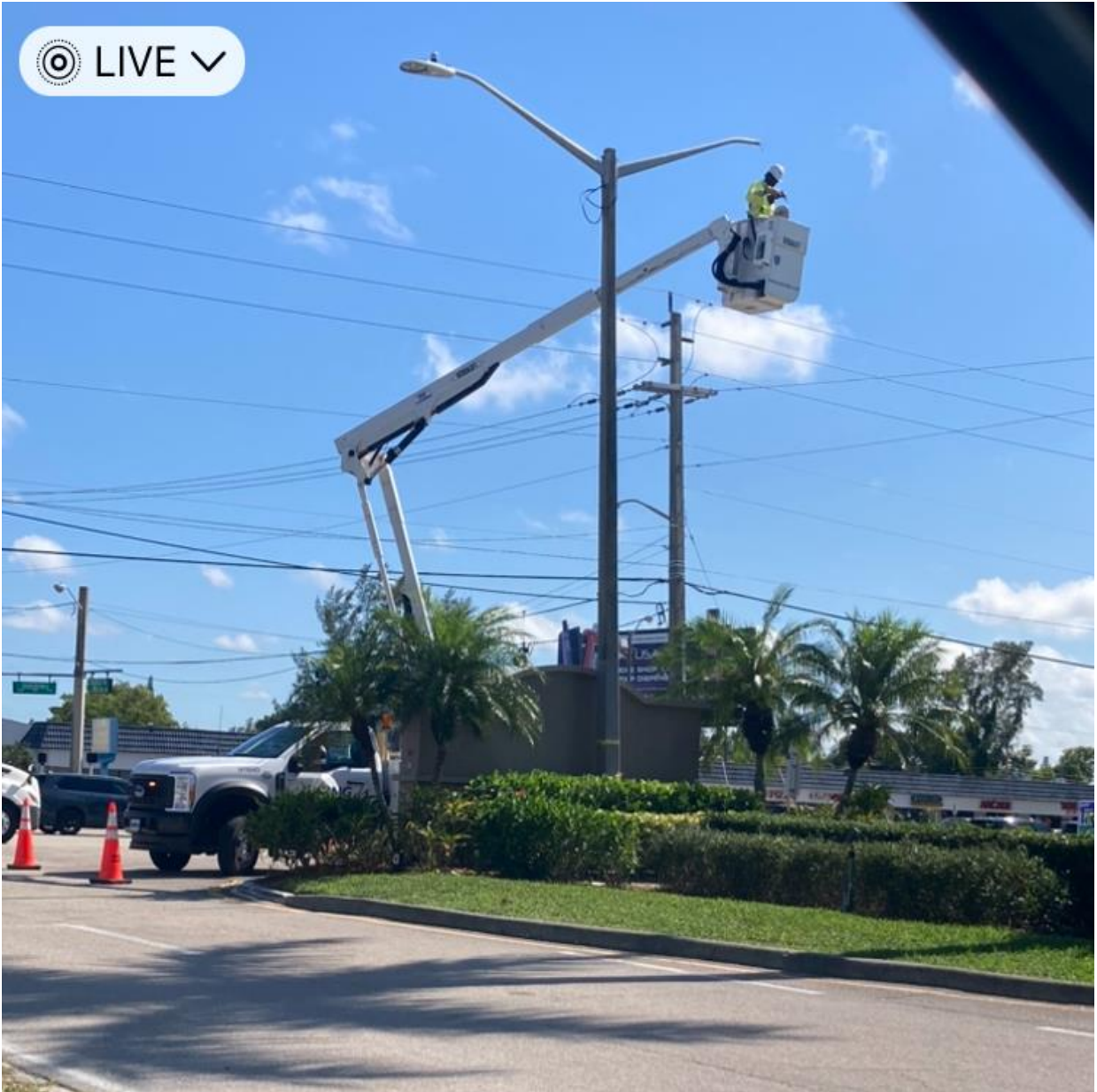
WEST DRIVE- LAST WEEK, FPL MADE REPAIRS TO STREET LIGHT FIXTURES AT WEST DRIVE, NORTH DRIVE, AND CENTURY BOULEVARD.
