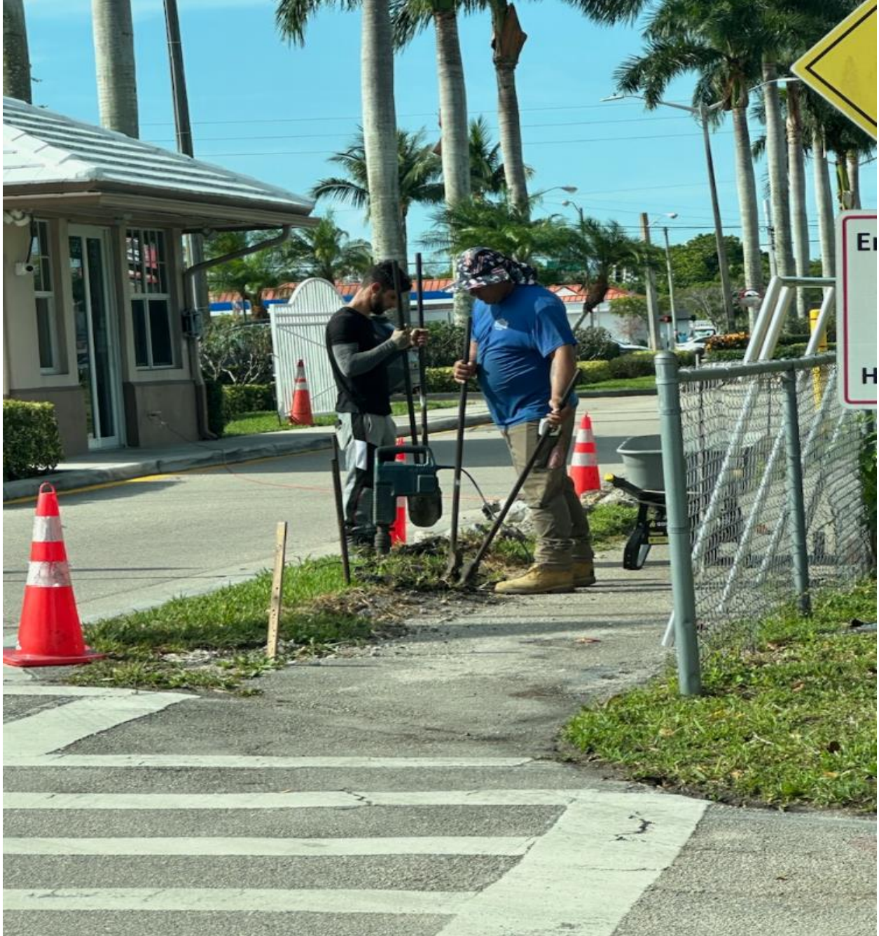
WEST DRIVE- ON 6/10, BUDGET FENCE AND GATE SYSTEMS REPLACED A RAILING ALONG A PEDESTRIAN WALKWAY.
