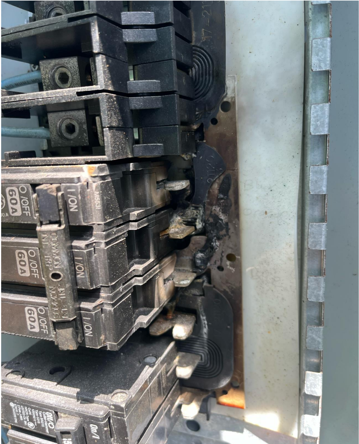
NORWICH IRRIGATION PUMP STATION- FRIED ELECTRICAL PANEL. T.S.I. ELECTRIC MADE REPAIRS AND IRRIGATION SERVICE WAS RESTORED TO THAT SECTION.
