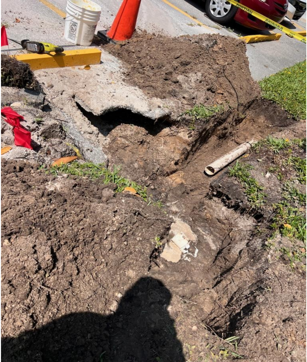
DORCHESTER C- THREE INCH IRRIGATION SUPPLY PIPE WAS REPAIRED BY SEACREST SERVICES.
