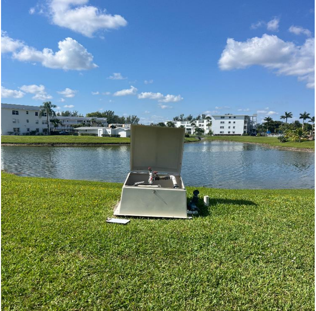
WELLINGTON H/J- SOME OF OUR SMALLER IRRIGATION PUMP STATIONS ARE COVERED BY FIBERGLASS "IGLOOS".
