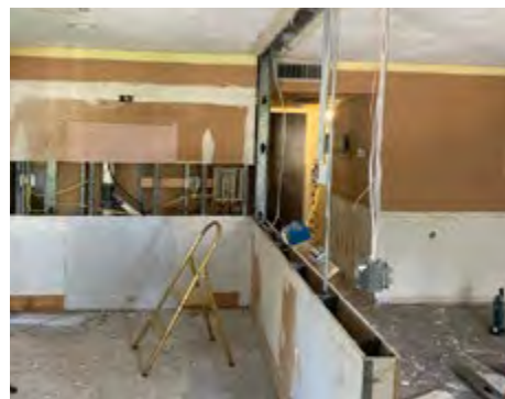
196 ANDOVER H- ANOTHER UNIT GUT JOB, INTERIOR WALLS REMOVED, NO PRIOR WRITTEN PERMISSION BY THE BOARD, NO PERMITS, SKETCHY ELECTRICAL WORK, INSUFFICIENT INSURANCE. NO GOOD. THIS BOARD ORDERED ALL WORK TO STOP AND WILL CONSULT WITH THEIR PROPERTY MANAGER AND ATTORNEY. A REPORT WAS SENT TO PBC CODE ENFORCEMENT, COMPLAINT #C-2024-06210005.
