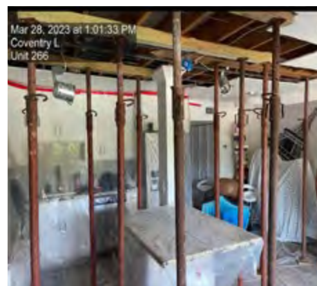
266 COVENTRY L- THIS IS WHAT CAN HAPPEN WHEN THE BOARD ALLOWS INTERIOR WALLS TO BE REMOVED WITHOUT PERMITS OR ENGINEERING. SECOND FLOORS COLLAPSE INTO FIRST FLOORS. NOT GOOD.
