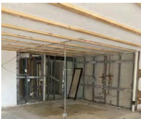
304 GREENBRIER B- HERE WE GO AGAIN. THIS UNIT OWNER TOLD THE PRESIDENT THAT THEY WERE REPLACING A SINK. SHE LEFT OUT THE PART ABOUT DESTROYING INTERIOR WALLS, REMOVING DRYWALL, INSTALLING RECESSED LIGHTING, INSTALLING A DROP CEILING, AND REROUTING ELECTRICAL LINES. EVERYBODY LIES. DON'T LET THIS HAPPEN TO YOU.
