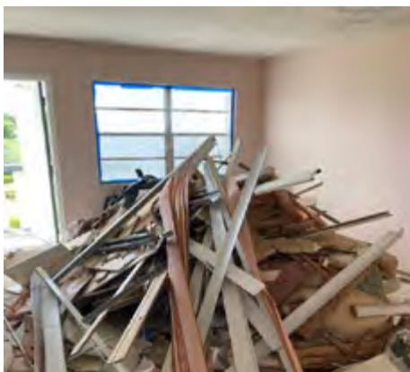
481 WELLINGTON K- THIS UNLICENSED CONTRACTOR PLANS TO DRAG EVERY BIT OF THIS JUNK DOWN FOUR FLIGHTS OF STAIRS. ASSOCIATIONS CAN REQUIRE DEPOSITS BEFORE WORK BEGINS, BUT THIS NEEDS TO BE IN THE ASSOCIATION'S DOCUMENTS.
