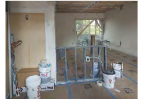
GOLFS EDGE 16A- THIS UNIT WAS RECENTLY GUTTED. THE BOARD DID GIVE PERMISSION, AND PERMITS WERE PULLED, BUT A CLOSE EXAMINATION OF THE INSURANCE CERTIFICATE SHOWED INADEQUATE WORKER'S COMP INSURANCE. WORK WAS STOPPED UNTIL THE INSURANCE IS STRAIGHTENED OUT. ALSO, THIS WORK VERY LIKELY NEEDED A MEMBERSHIP VOTE BEFORE THE WORK WAS AUTHORIZED BY THE BOARD. CHECK WITH YOUR ASSOCIATION'S ATTORNEY BEFORE APPROVING CONSTRUCTION PROJECTS.
