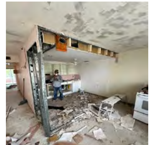
481 WELLINGTON K- INTERIOR WALLS DESTROYED. NO PERMISSION FROM THE BOARD, NO PERMIT, NO EVIDENCE OF CONTRACTOR INSURANCE OR LICENSURE. NO GOOD. REPORTED TO PBC CODE ENFORCEMENT, COMPLAINT #C-2024-06240001.
