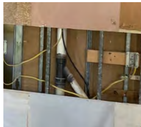
196 ANDOVER H- YIKES! CUT PIECES OF EXTENSION CORDS USED AS ELECTRICAL WIRING. A FIRE WAITING TO HAPPEN.
