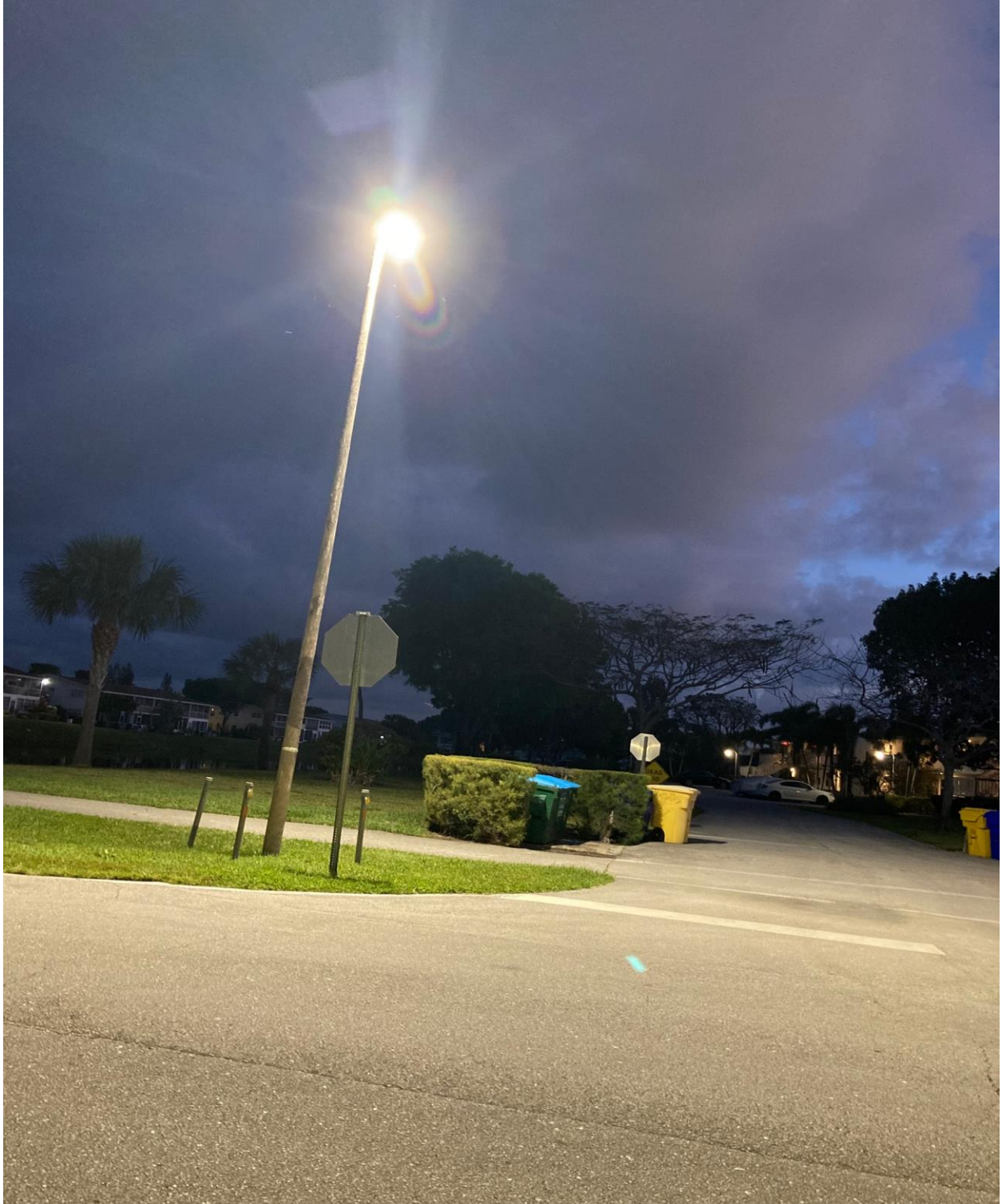
SOUTH DRIVE- THIS STREETLIGHT IS MAINTAINED BY UCO, AND WAS RECENTLY REPAIRED BY SEACREST SERVICES.
