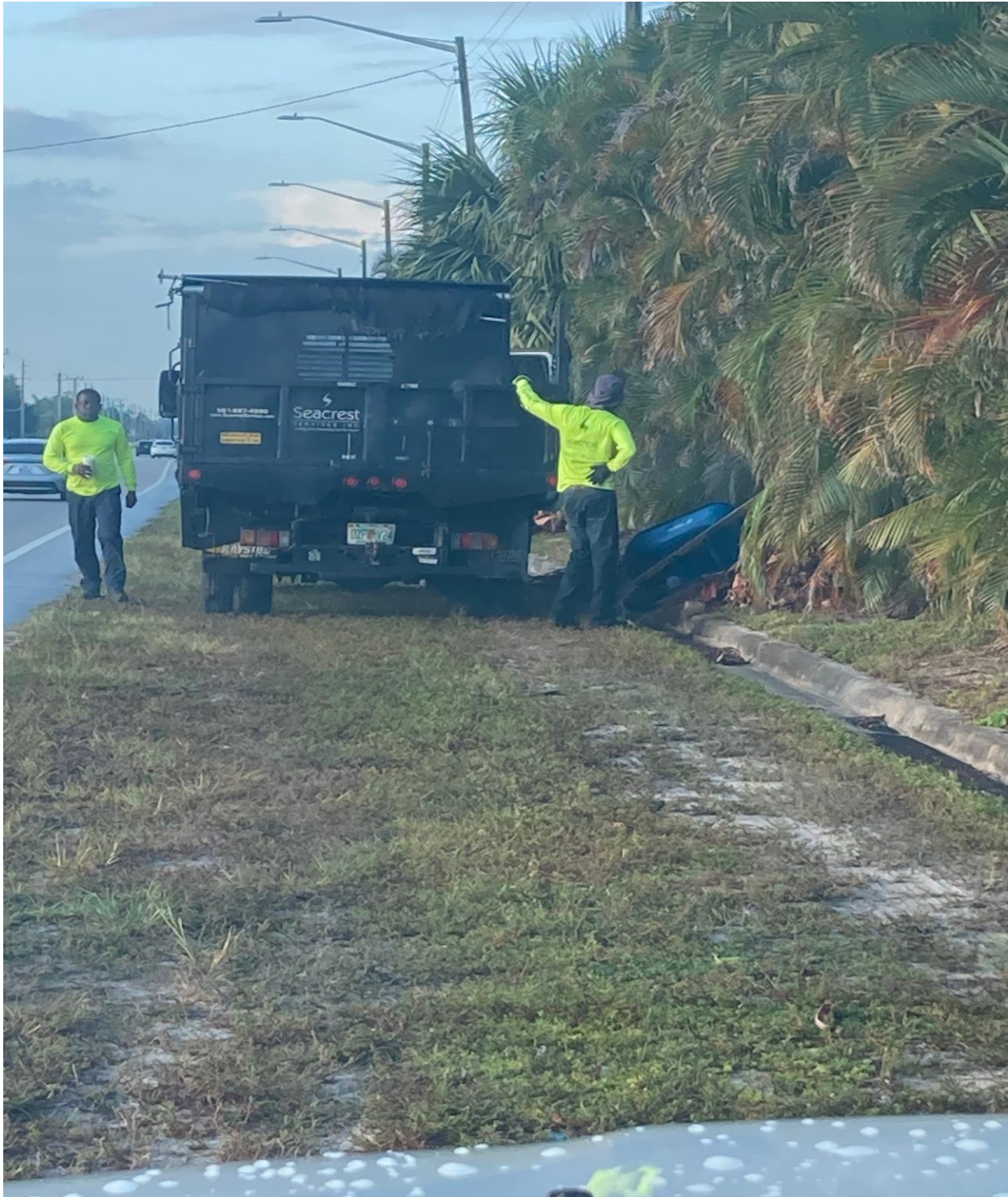
HAVERHILL ROAD- ON 4/30, SEACREST SERVICES PERFORMED QUARTERLY CLEANUP OF THE GRASS SWALE AND ARECA PALM HEDGE. CLEARING DEAD PALM FRONDS FROM UNDER THE ARECAS REDUCES RAT ACTIVITY IN THE AREA.
