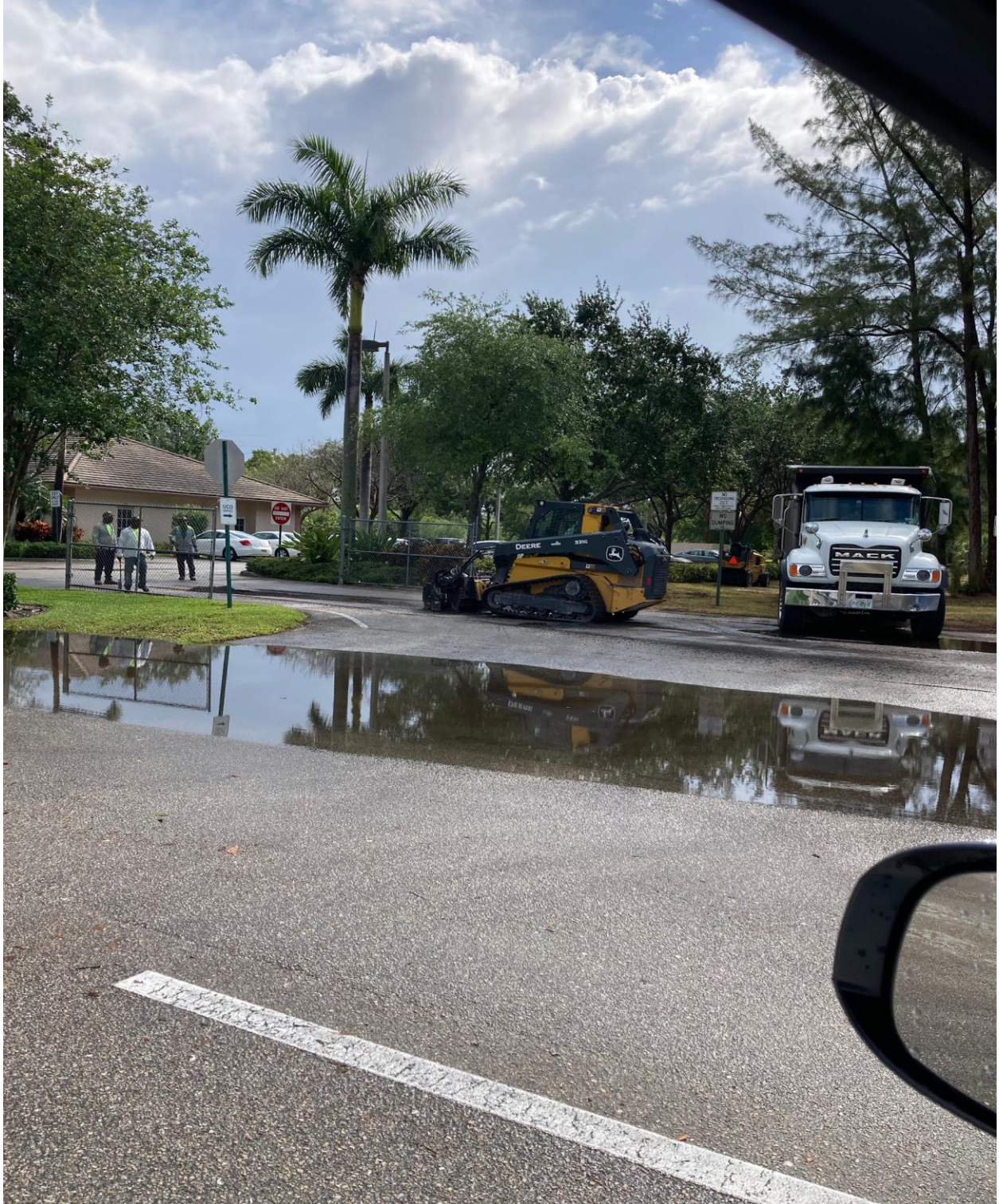
UCO OFFICE- LAST WEEK, SUNSHINE PAVING PERFORMED ROAD AND WALKWAY REPAIRS AT VARIOUS SECTIONS OF CV.
