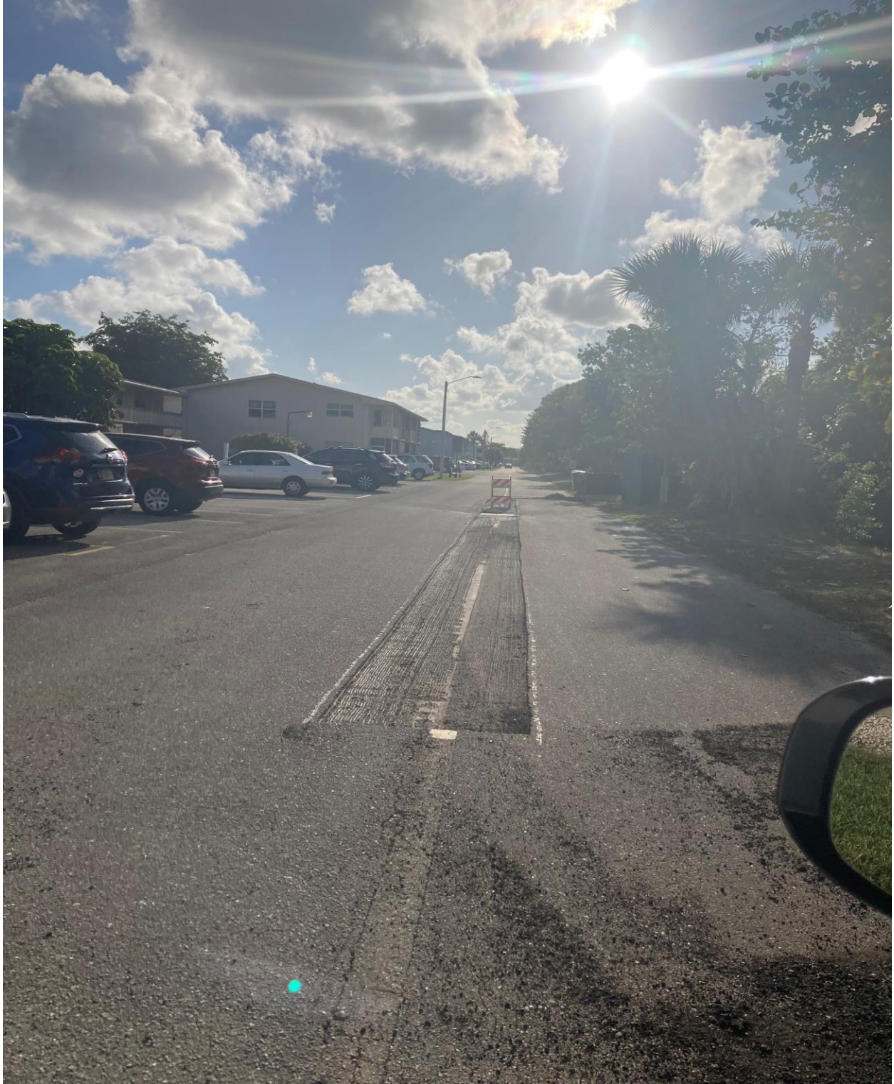
FALKIRK STREET- DETERIORATED SECTION OF ROAD WAS PREPARED ON 5/2. REPAIR WAS COMPLETED ON 5/3.
