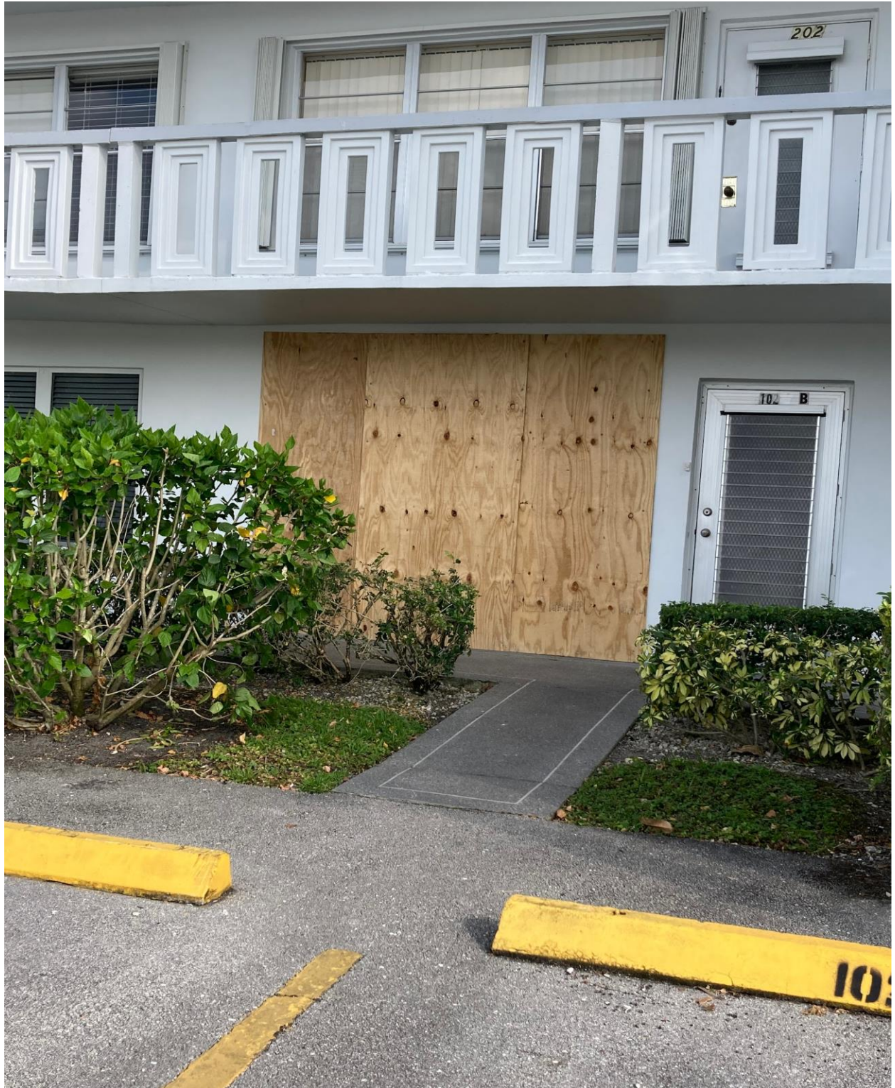
102 WELLINGTON B- CR1 HOME AND REMODELING GOT RIGHT OVER TO BOARD UP THE DAMAGED AREA.
