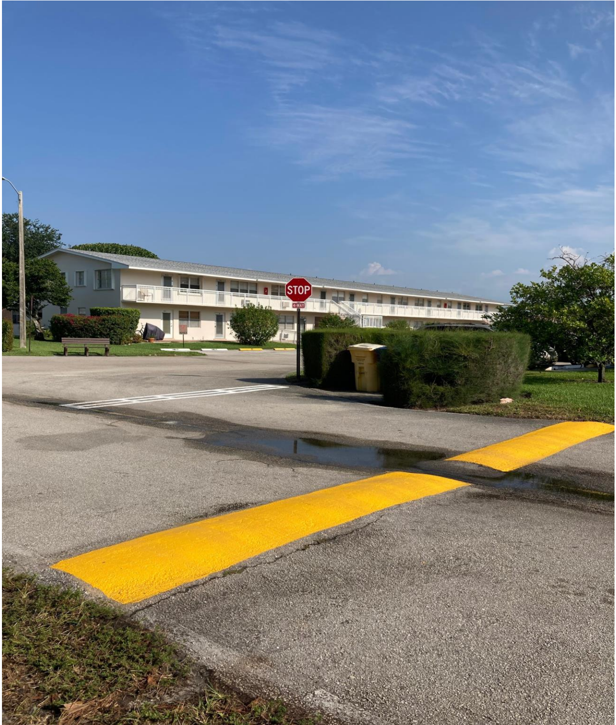
HASTINGS SECTION- JOSE PAINTED SPEED BUMPS AND STOP BARS ON SATURDAY, 5/18. THIS WILL BE AN ONGOING PROJECT.
