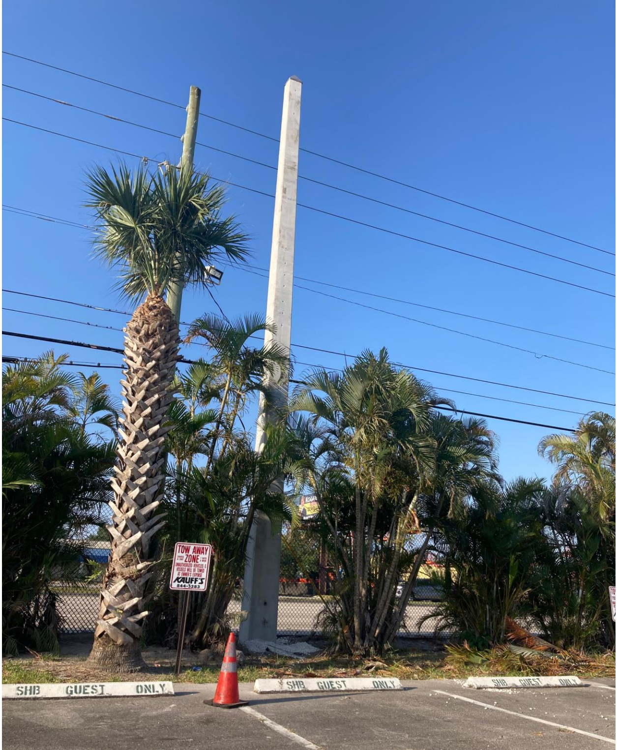
SOUTHAMPTON SECTION- FPL INSTALLED NEW CONCRETE UTILITY POLES ALONG THE OKEECHOBEE BOULEVARD FENCE.
