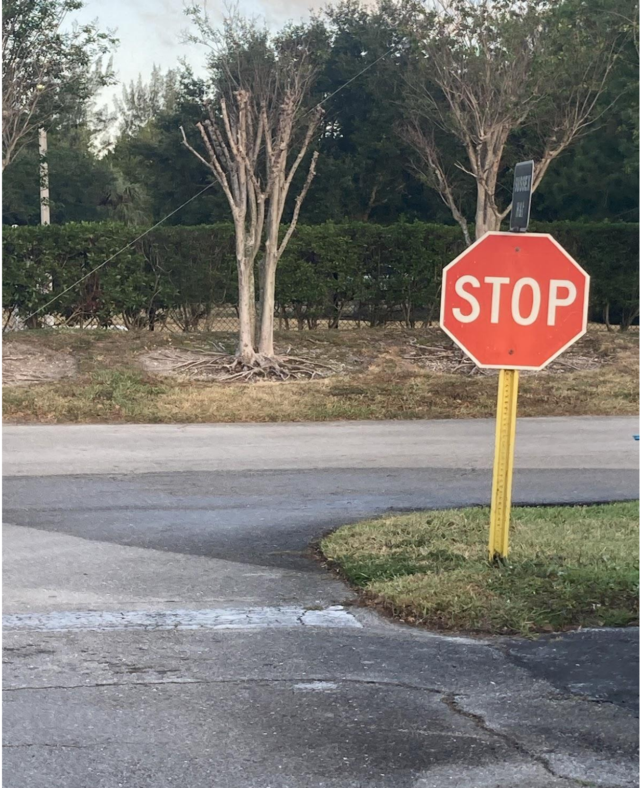
SUSSEX SECTION- THIS MIDGET STOP SIGN IS FADED AND TOO SHORT, AND THE STOP BAR NEEDS TO BE REPAINTED WITH FDOT COMPLIANT TRAFFIC PAINT.
