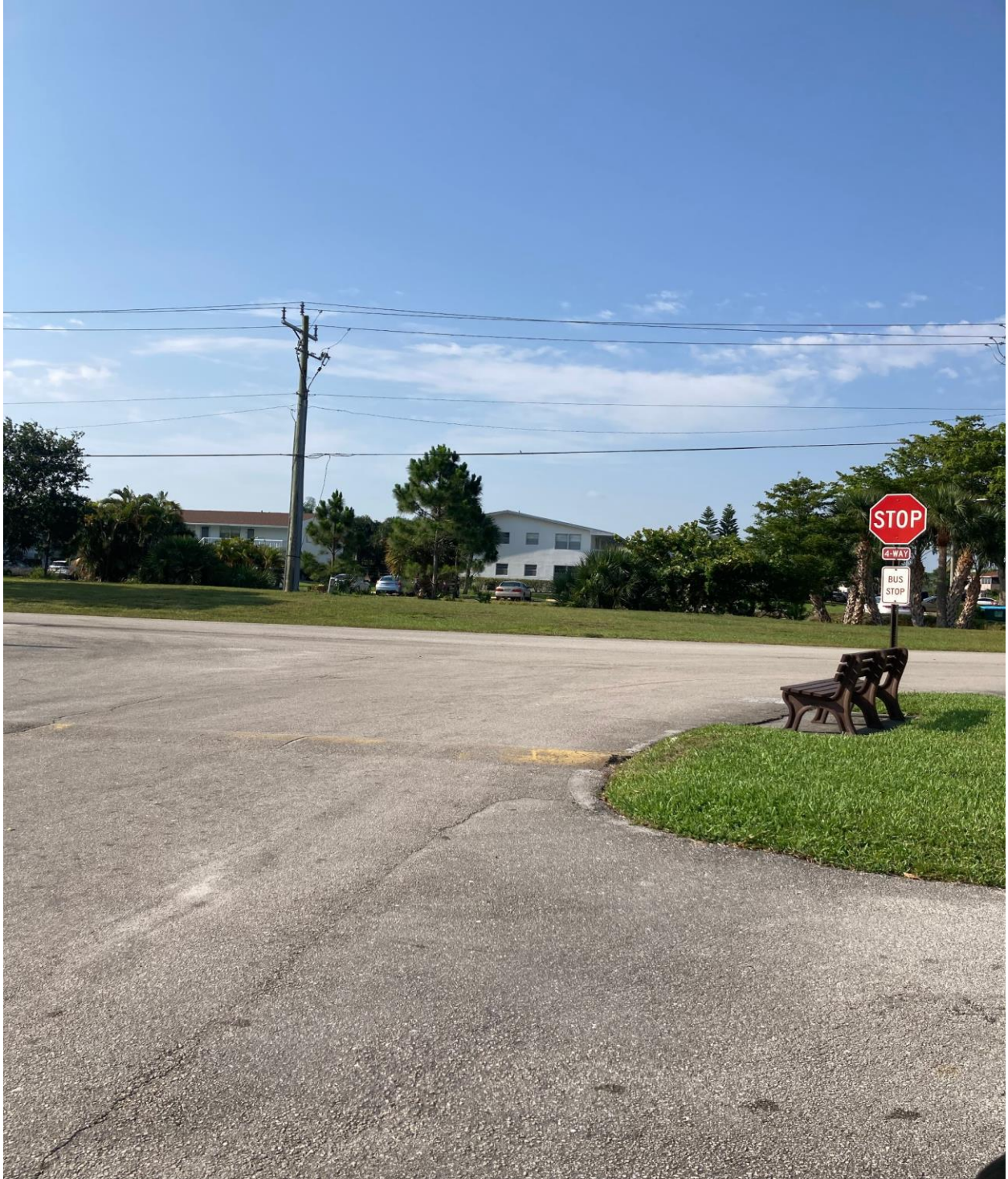
HASTINGS SECTION- AT MANY OF THE SECONDARY/TERTIARY ROAD INTERSECTIONS, SPEED BUMP AND STOP BAR PAINT HAS NEARLY DISAPPEARED.
