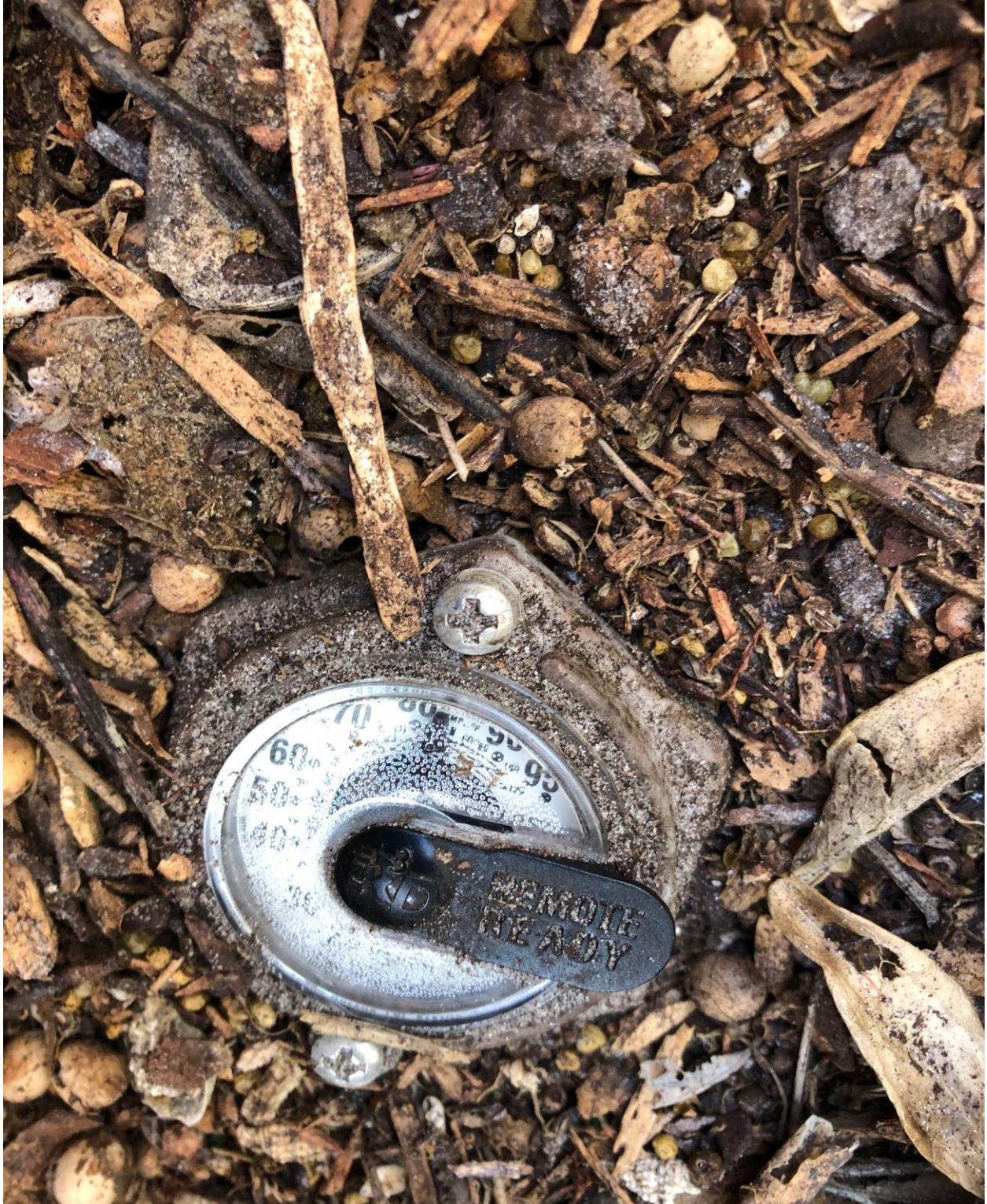
OKEECHOBEE BOULEVARD GUARDHOUSE- PROPANE FUEL TANK FOR EMERGENCY GENERATOR- APPROXIMATELY 400 GALLONS.
