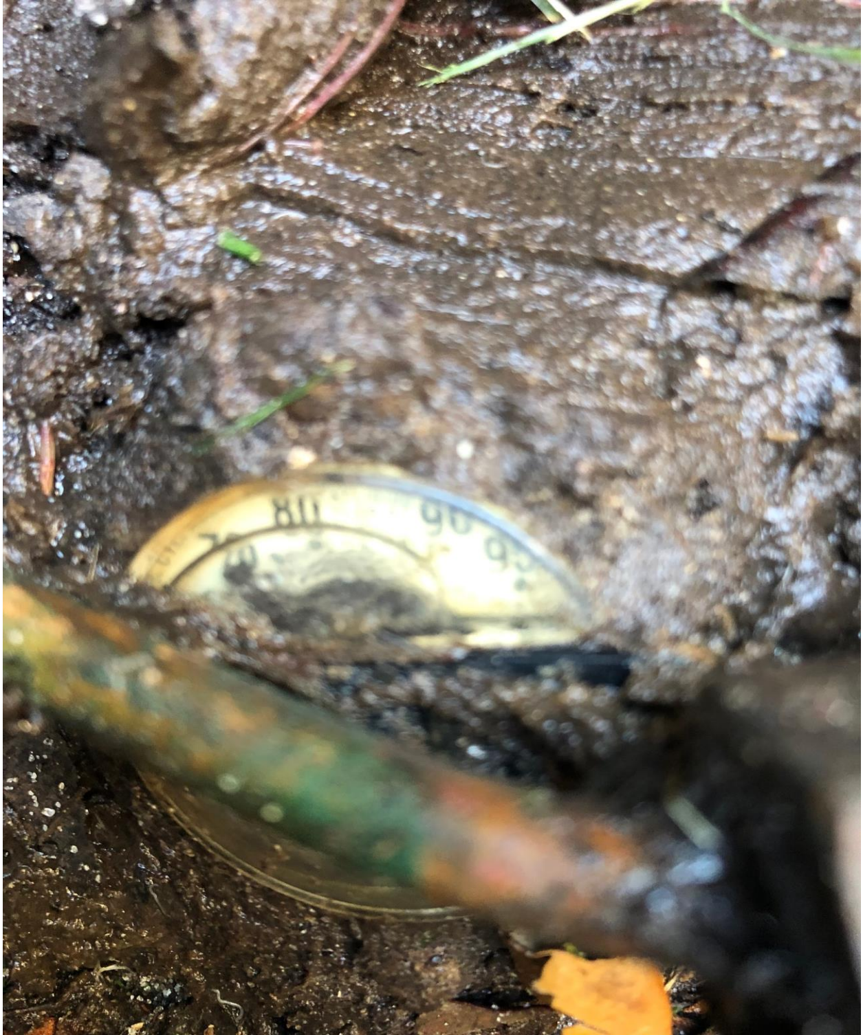
UCO OFFICE- PROPANE FUEL TANKS FOR EMERGENCY GENERATOR- APPROXIMATELY 700 GALLONS.
