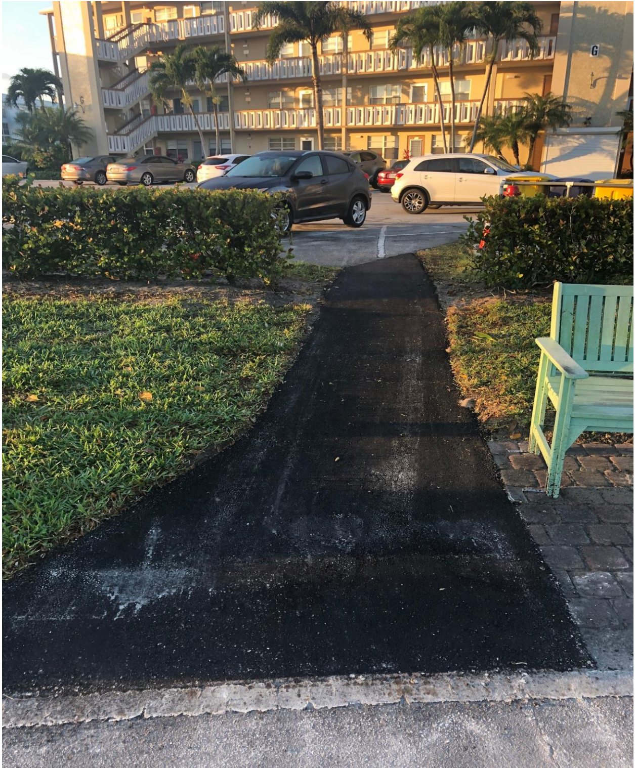
WELLINGTON G- A ROOT DAMAGED WALKWAY WAS REPAIRED BY ATLANTIC SOUTHERN PAVING.
