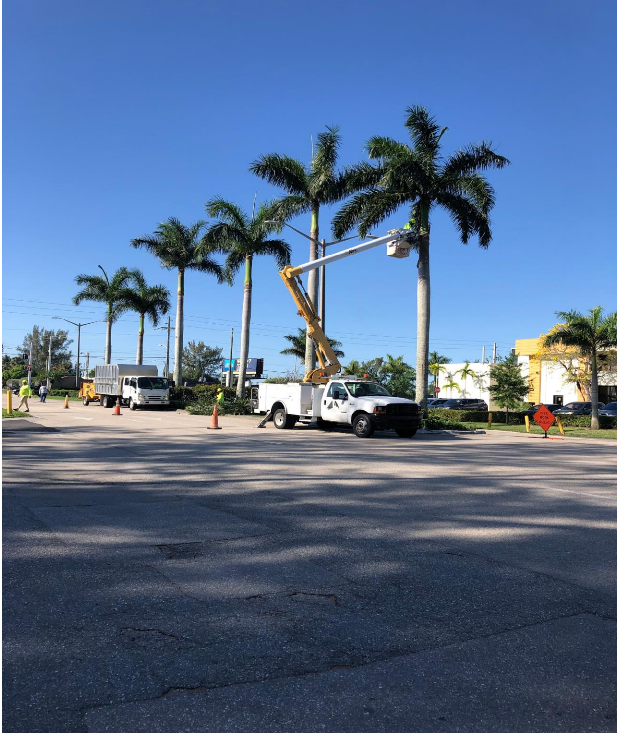
WEST DRIVE- ON 3/29, REQUELME TREE SERVICE BEGAN ANNUAL MAINTENANCE TRIM OF TREES AND PALMS ON UCO OWNED AND MAINTAINED PROPERTY. THIS WORK WILL CONTINUE NEXT WEEK.
