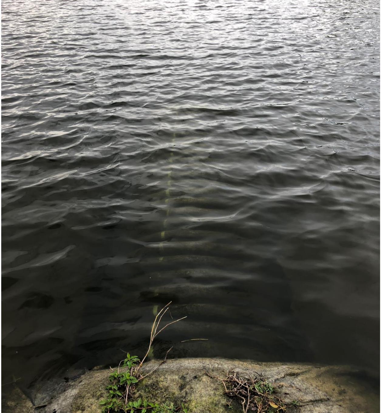
STRATFORD D- THIS IS THE RECENTLY RELINED DRAIN PIPE THAT RUNS UNDER THE DIP IN THE GRASS.
