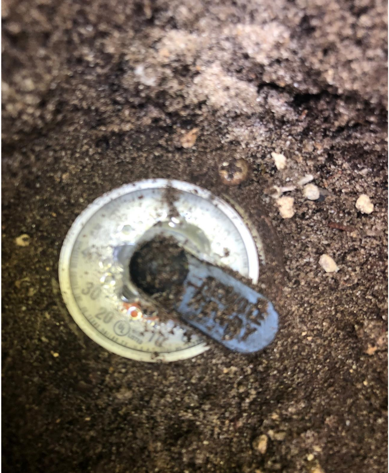
HAVERHILL ROAD GUARDHOUSE- PROPANE FUEL SUPPLY FOR EMERGENCY GENERATOR CONFIRMED, 350 GALLONS.
