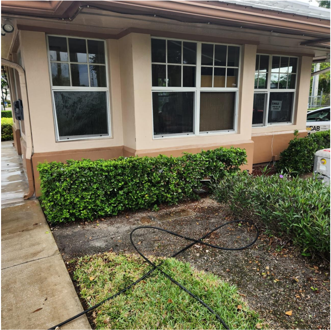
OKEECHOBEE BOULEVARD GUARDHOUSE- THESE BUILDING EXTERIORS GET GRIMY AND NEED TO BE WASHED PERIODICALLY.
