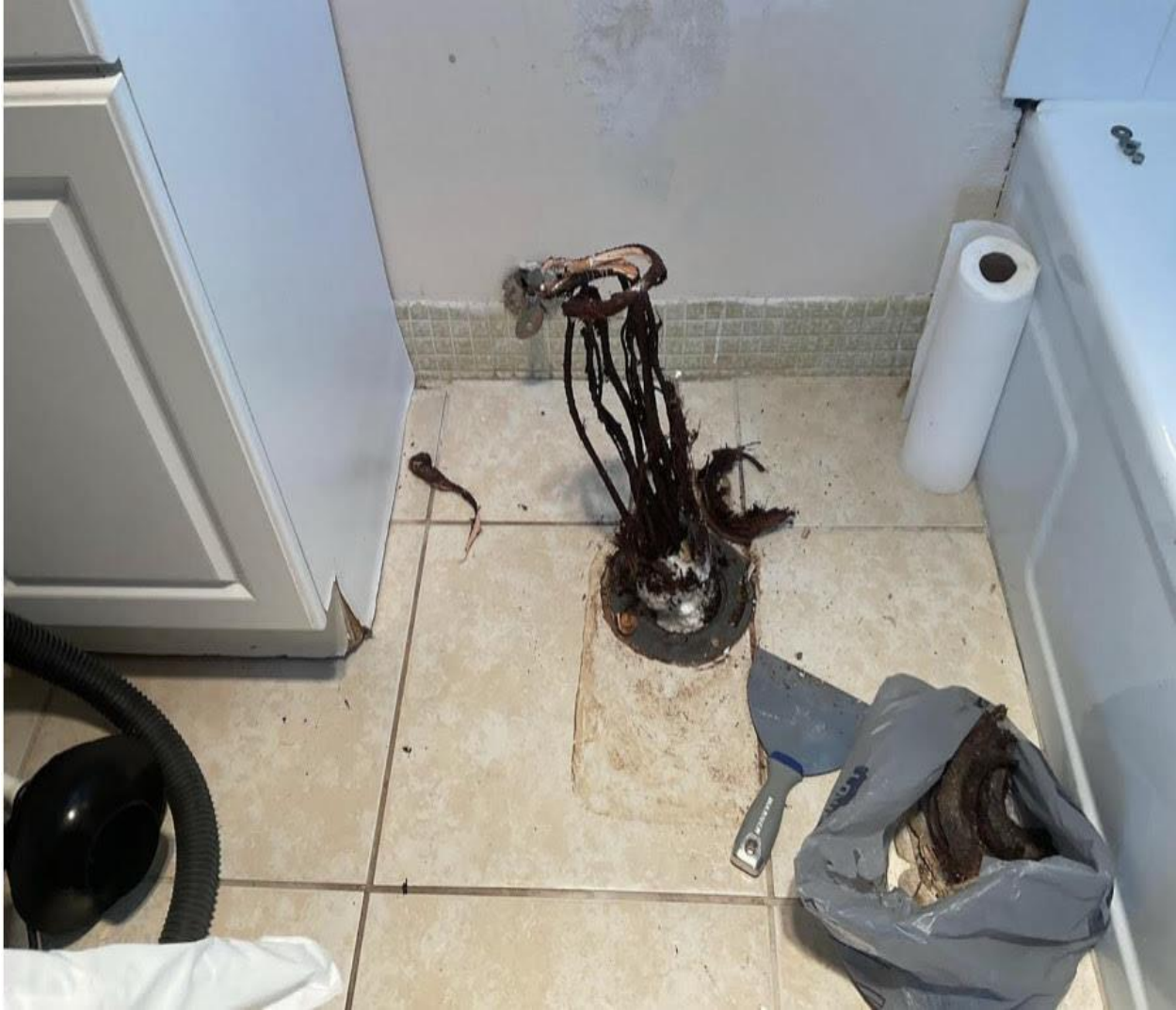
TOILET TREE- THIS IS ALWAYS AN UNPLEASANT SURPRISE AT A PLACE AND TIME THAT A UNIT OWNER IS LEAST LIKELY TO APPRECIATE IT.
