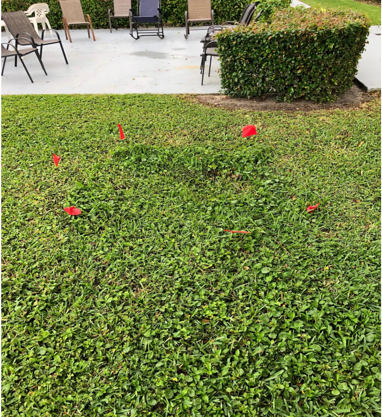
STRATFORD D- THIS DIP IN THE GRASS WAS RIGHT ON TOP OF A RECENTLY RELINED STORM WATER DRAINAGE PIPE.
