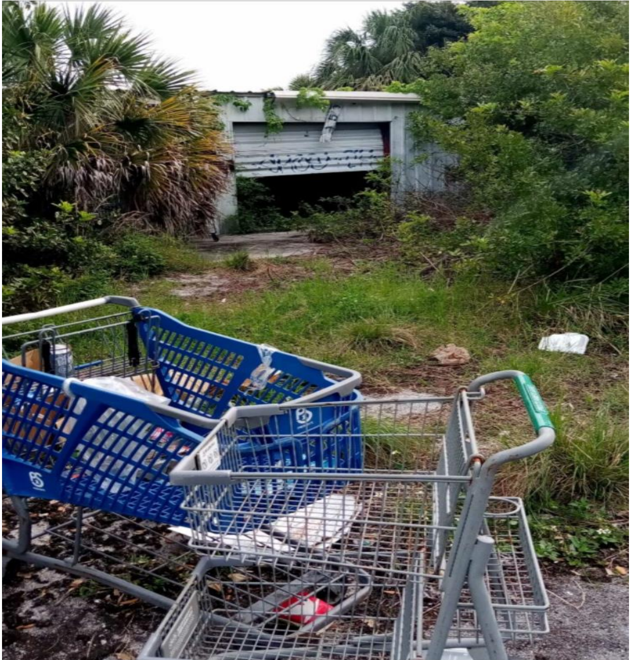
REFLECTION BAY- THIS DISUSED GARAGE BUILDING, NEAR THE CV/RB PROPERTY LINE, IS BEING USED BY HOMELESS PERSONS FOR SHELTER. NOTE THE SPRAY PAINTED MARKINGS ON THE GARAGE DOOR.
