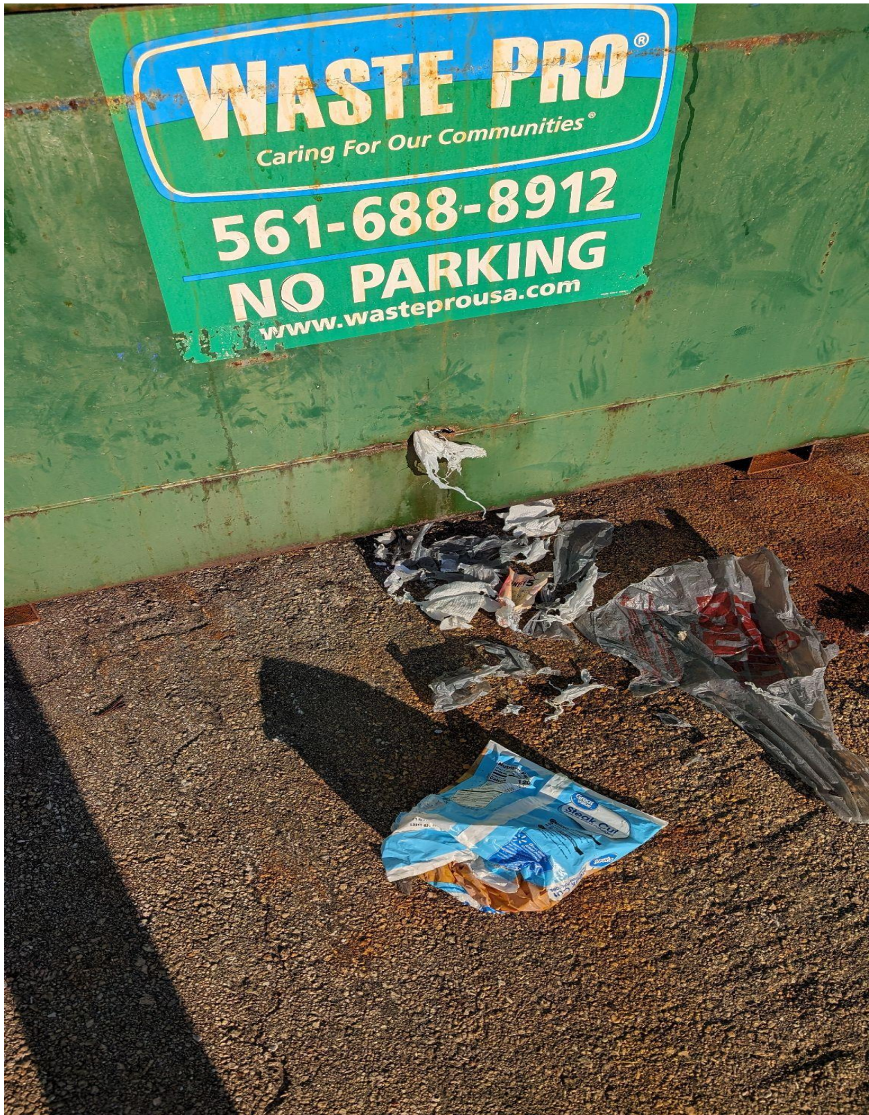
SUSSEX A- RUSTED OUT DUMPSTER. REPORTED IN BY A CV UNIT OWNER. REQUEST FOR REPLACEMENT WAS SENT TO WASTE PRO.
