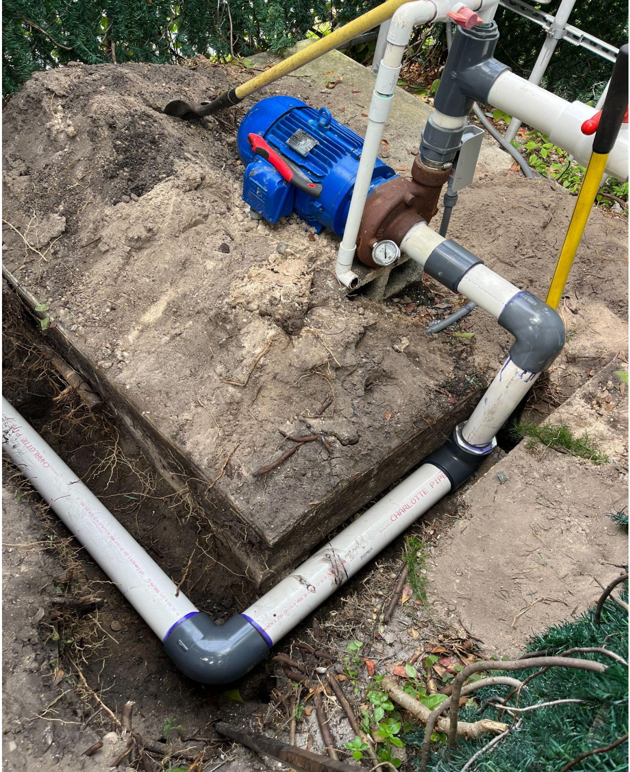
STRATFORD SECTION- LAST WEEK. AN UNDERGROUND PIPE LEAK AT THIS IRRIGATION PUMP STATION WAS EXCAVATED BY SEACREST SERVICES AND REPAIRED BY CHABOT IRRIGATION.
