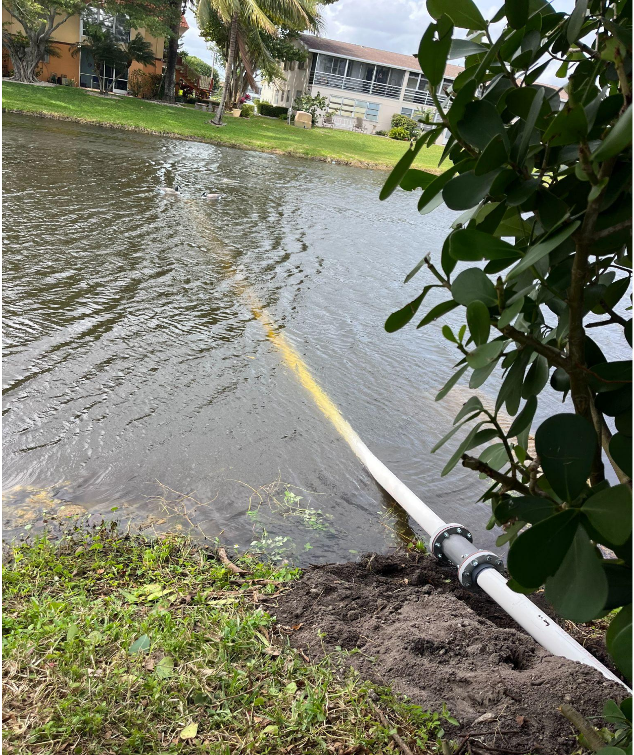
SHEFFIELD SECTION- NEW IRRIGATION INTAKE PIPE, WITH NEW SCREENS AND NEW CHECK VALVE, INSTALLED BY CHABOT IRRIGATION ON 3/5.
