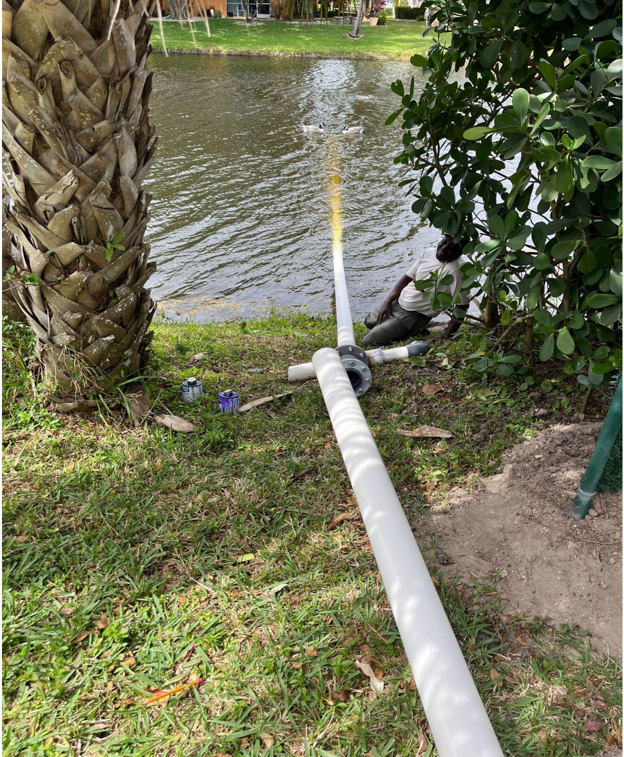
SHEFFIELD SECTION- THIS IRRIGATION INTAKE PIPE WAS REPLACED BY CHABOT IRRIGATION ON 3/5.
