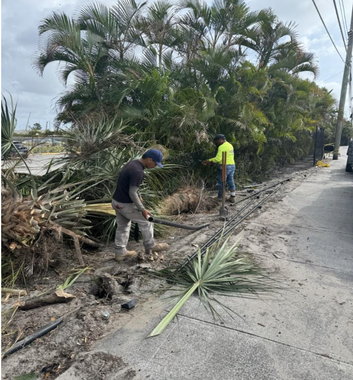
OKEECHOBEE BOULEVARD- BUDGET GATE AND FENCE MADE TEMPORARY REPAIRS TO THE FENCE ON SATURDAY, 3/2.
