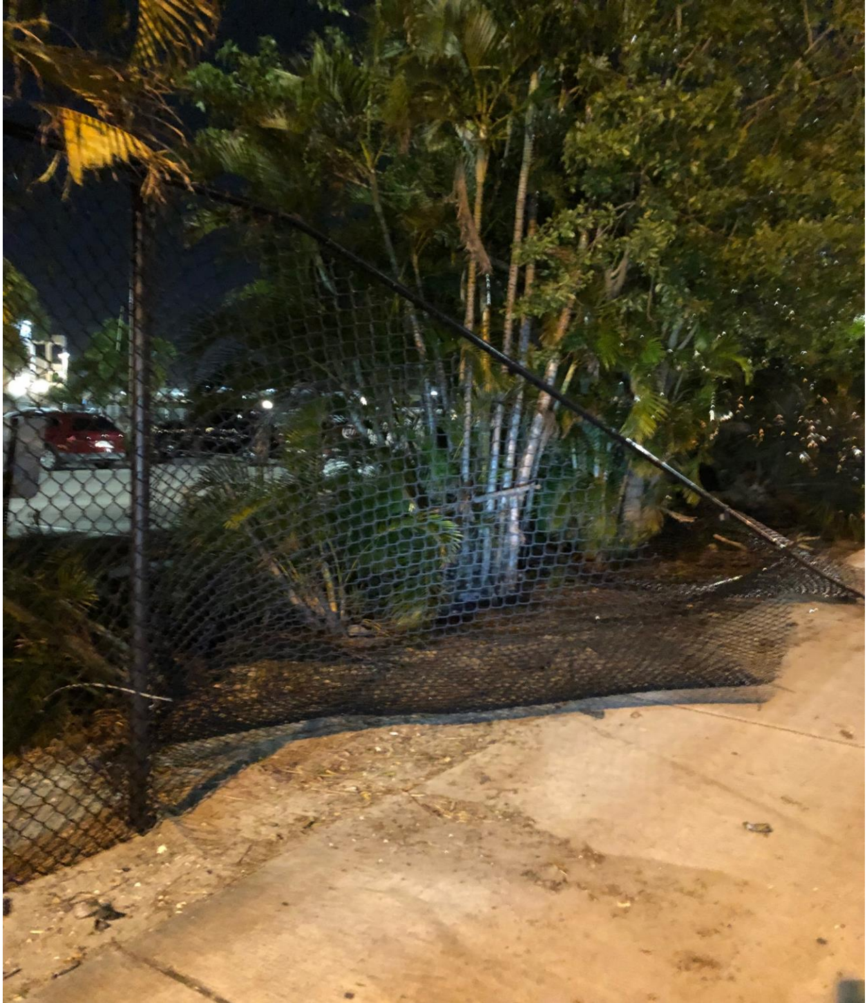
OKEECHOBEE BOULEVARD- THIS WRECKED OUT FENCE WILL BE PERMANENTLY REPAIRED AS SOON AS POSSIBLE.
