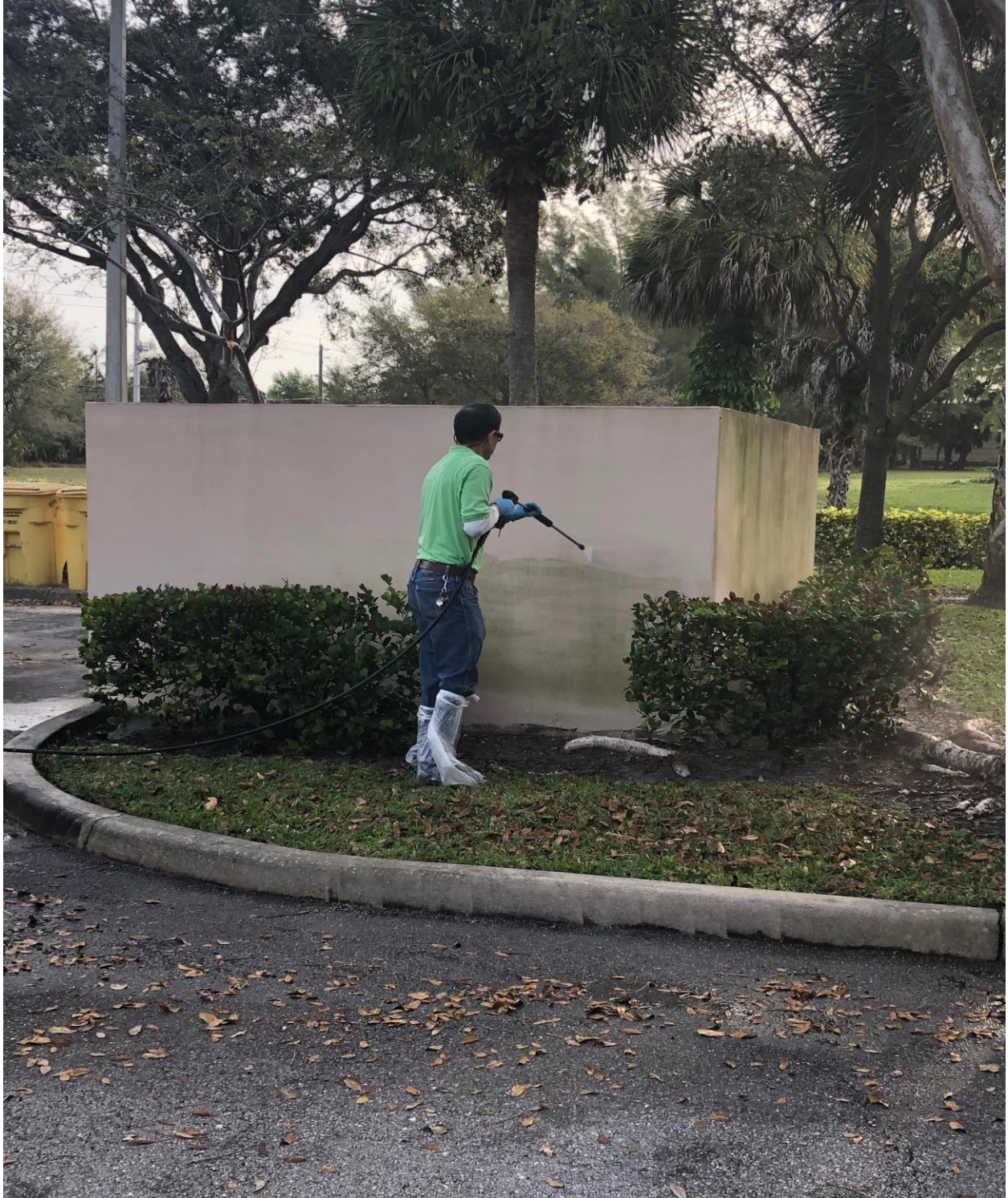
UCO OFFICE- EXTERIOR WALLS, WALKWAYS AND CURBS WERE PRESSURE CLEANED BY GLOW CLEANING PLUS ON 3/2.
