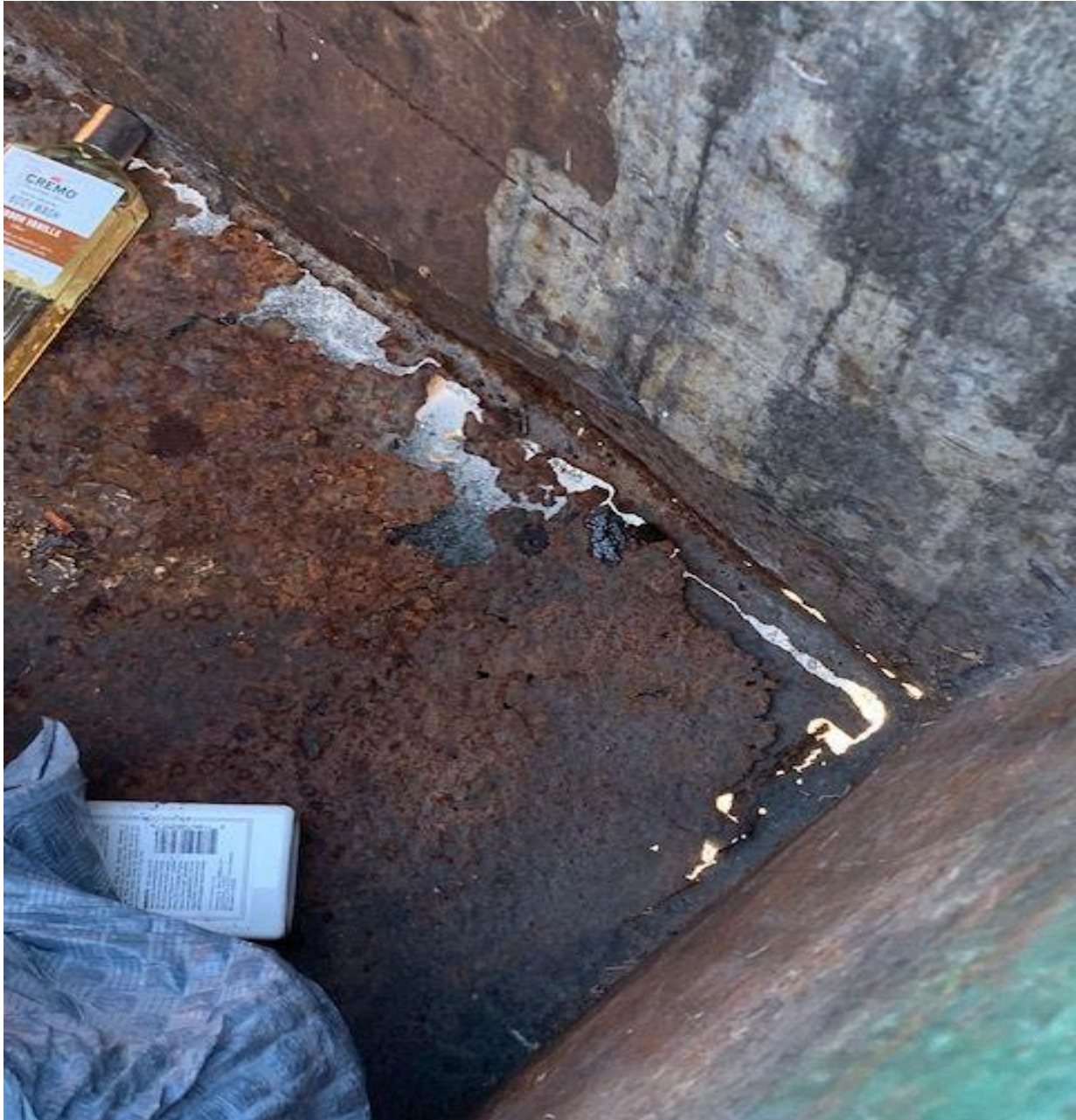
SOMERSET B- ROTTED OUT DUMPSTER, REPORTED IN BY A CV UNIT OWNER. REQUEST FOR REPLACEMENT WAS SENT TO WASTE PRO.
