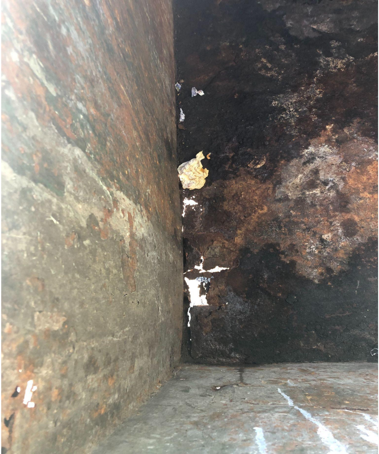
BEDFORD B- RUSTED OUT DUMPSTER. A REQUEST FOR REPLACEMENT WAS SENT TO WASTE PRO.
