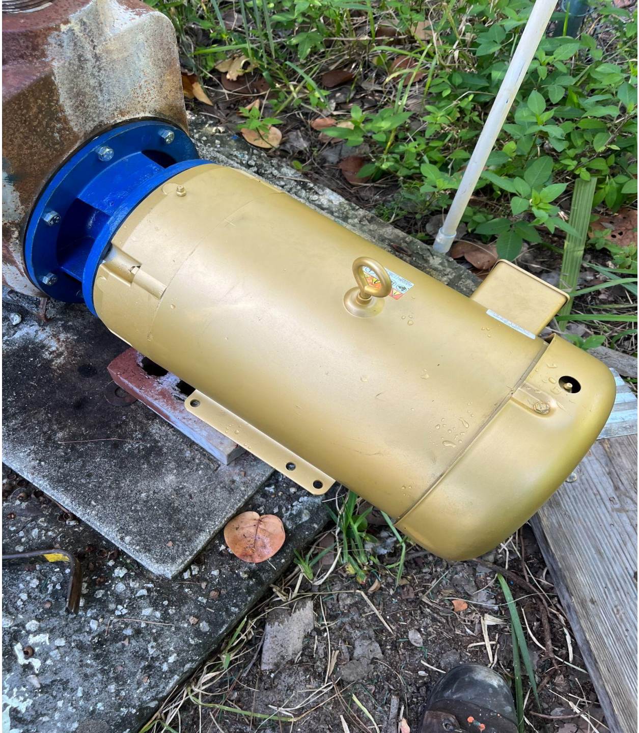
COVENTRY SECTION- NEW BALDOR PUMP MOTOR INSTALLED BY CHABOT IRRIGATION ON 2/7.
