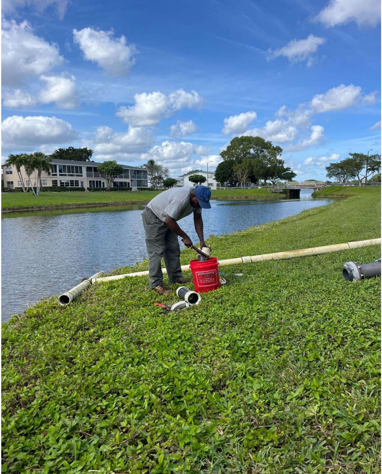
SOUTH LAGOON- INTAKE PIPE FOR THE BEDFORD SECTION IRRIGATION PUMP STATION WAS PULLED OUT AND REPAIRED BY CHABOT IRRIGATION ON 2/6.
