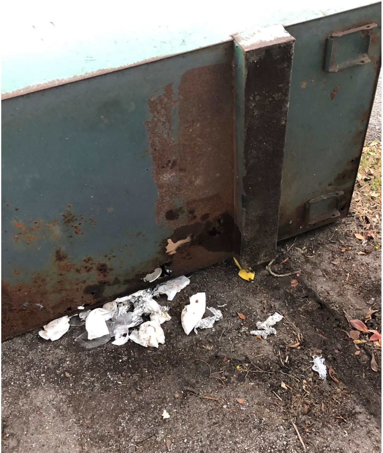
SHEFFIELD P- RUSTED OUT DUMPSTER. REQUEST FOR REPLACEMENT WAS SENT TO WASTE PRO.
