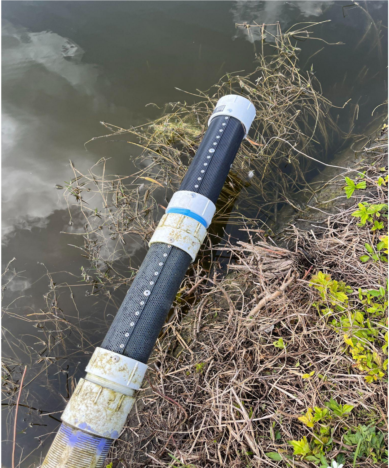
BEDFORD SECTION- NEW INTAKE SCREENS INSTALLED ON LAGOON END OF PUMP INTAKE PIPE. THESE KEEP MUD AND JUNK OUT OF THE PUMP.
