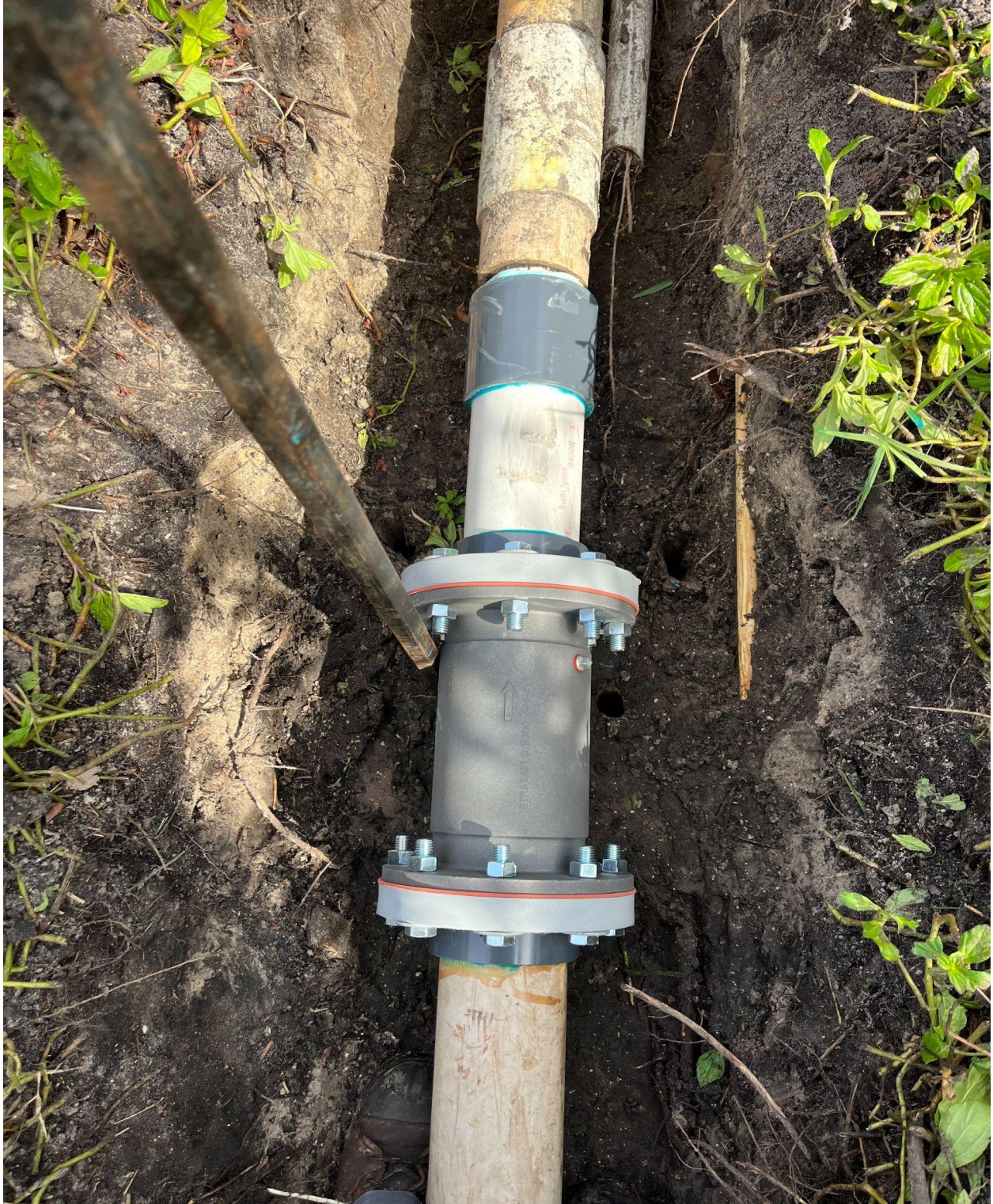
BEDFORD SECTION- NEW CHECK VALVE INSTALLED AT PUMP STATION INTAKE LINE. THIS VALVE KEEPS WATER RUNNING IN ONE DIRECTION, FROM THE LAGOON TO THE PUMP.
