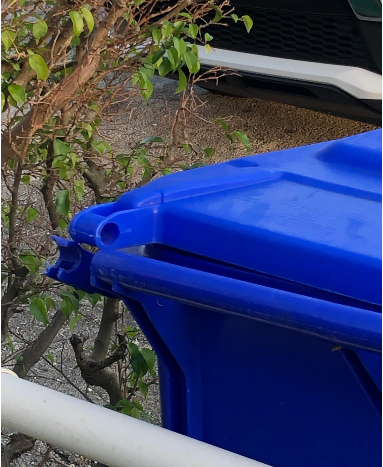
KENT B- BUSTED LID, BLUE TOTER. CALLED IN BY A CV UNIT OWNER. REQUEST FOR REPAIR WAS SENT TO WASTE PRO.
