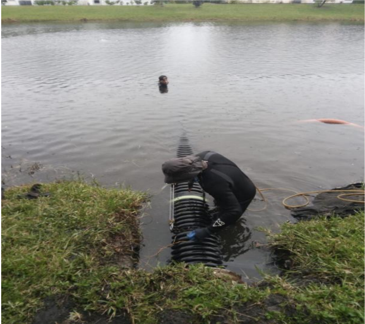
OXFORD SECTION- THIS ROTTED OUT SECTION OF STORM DRAIN PIPE WAS REPAIRED AND RELINED BY ANCHOR MARINE ON 1/2/24.
