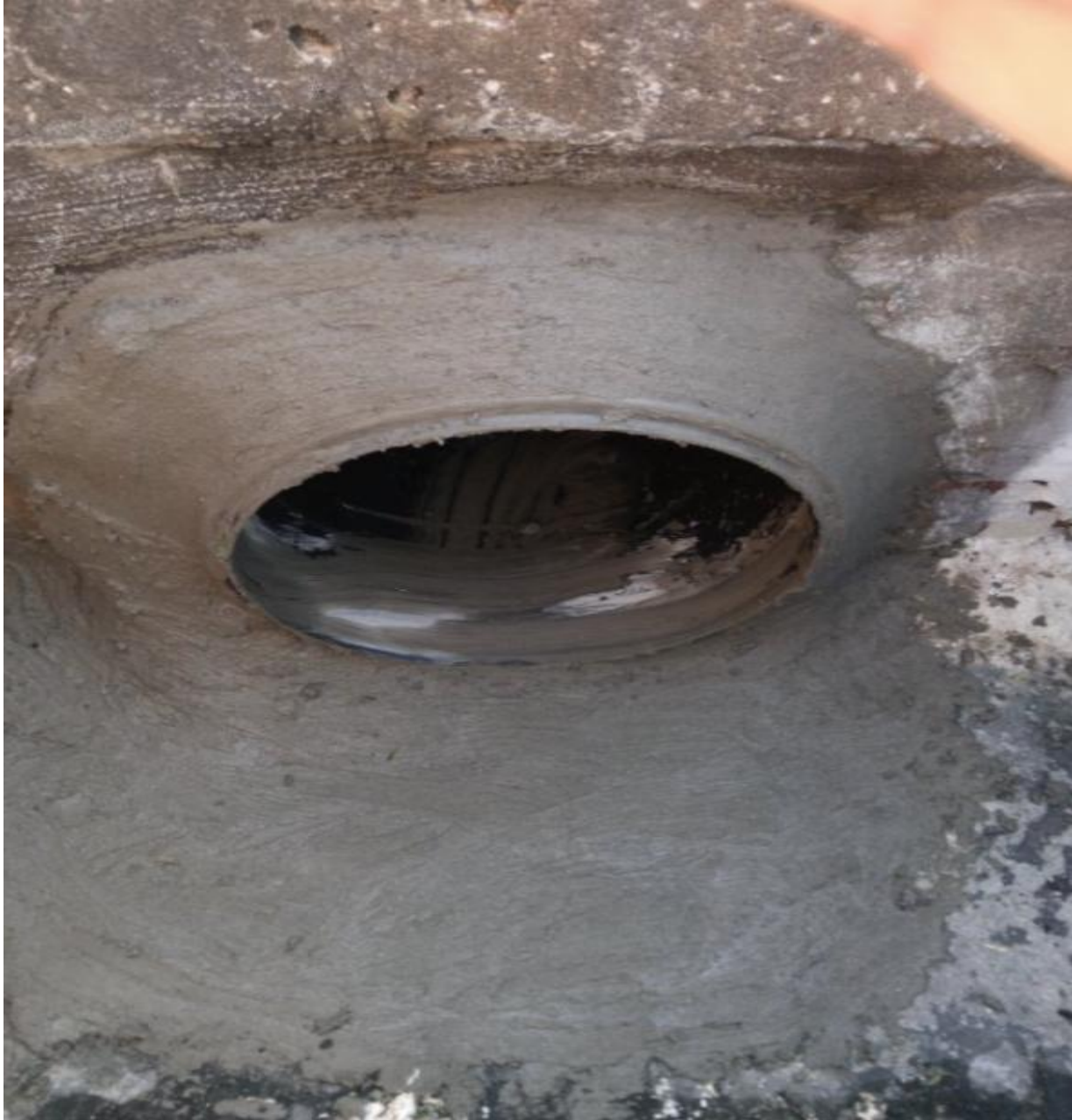
OXFORD SECTION- THIS IS THE OTHER END OF THE RELINED PIPE, GROUTED IN PLACE INSIDE OF A STORM WATER CATCH BASIN.
