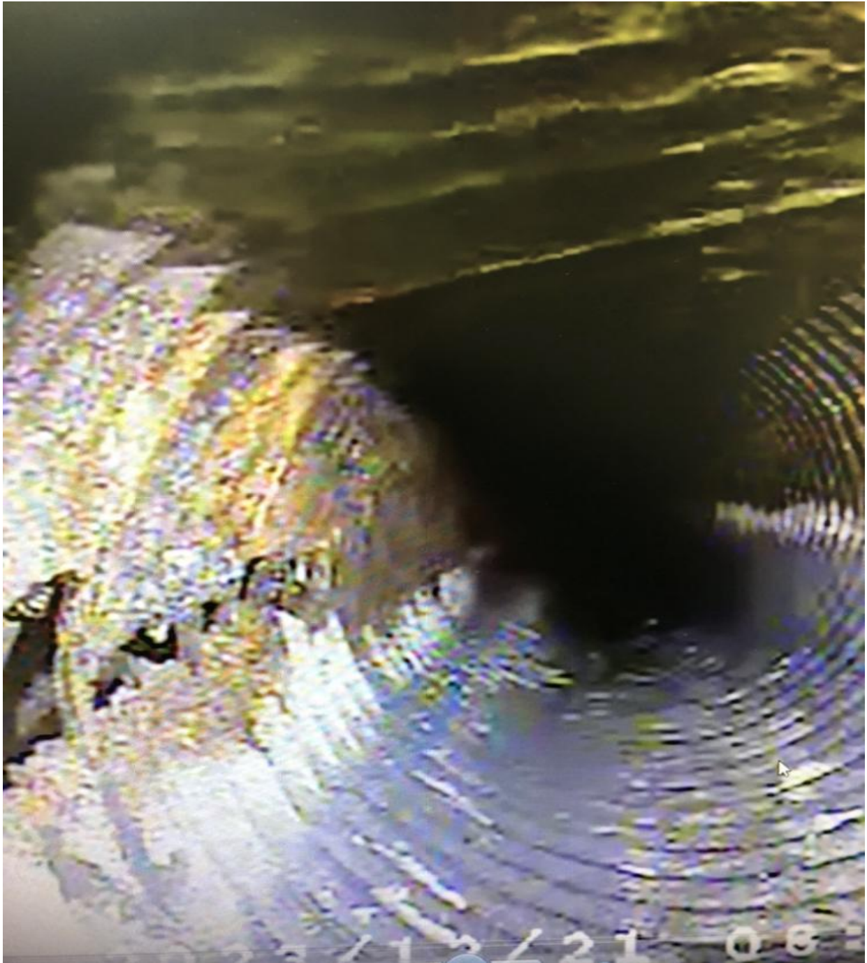
OXFORD SECTION- THIS UNDERGROUND STORM DRAIN PIPE WAS FOUND TO BE DAMAGED.
