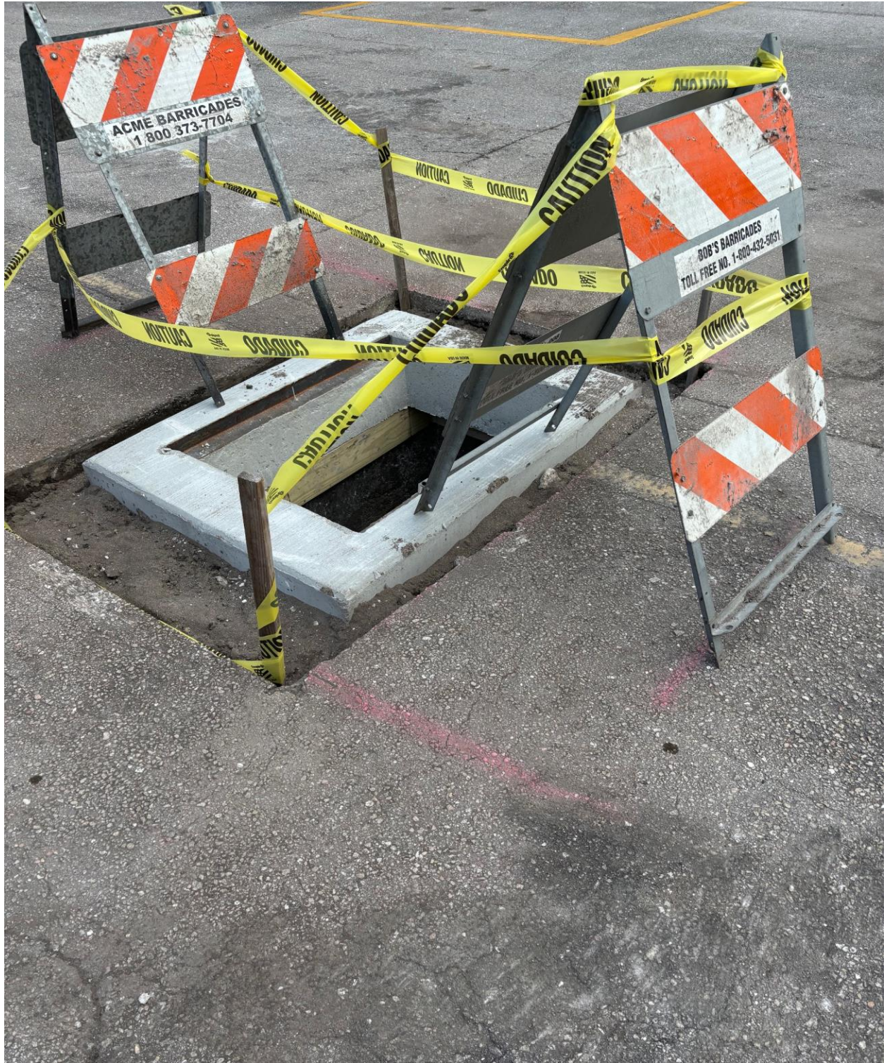
SHEFFIELD SECTION- ATLANTIC SOUTHERN PAVING INSTALLED NEW CATCH BASINS, REPLACING ORIGINAL BASINS WHICH HAD SUNK BELOW THE ROAD.
