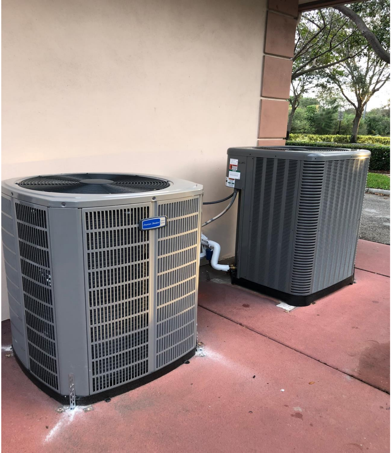
UCO OFFICE- NEW AC CONDENSER, ON LEFT, WAS INSTALLED BY AC ALL STARS ON 1/26. THE CONDENSER ON THE RIGHT IS SLIGHTLY LARGER BECAUSE IT COOLS THE FRONT HALF OF THE BUILDING, WHICH HAS A FRONT ENTRY DOOR OPENING AND CLOSING ALL DAY.
