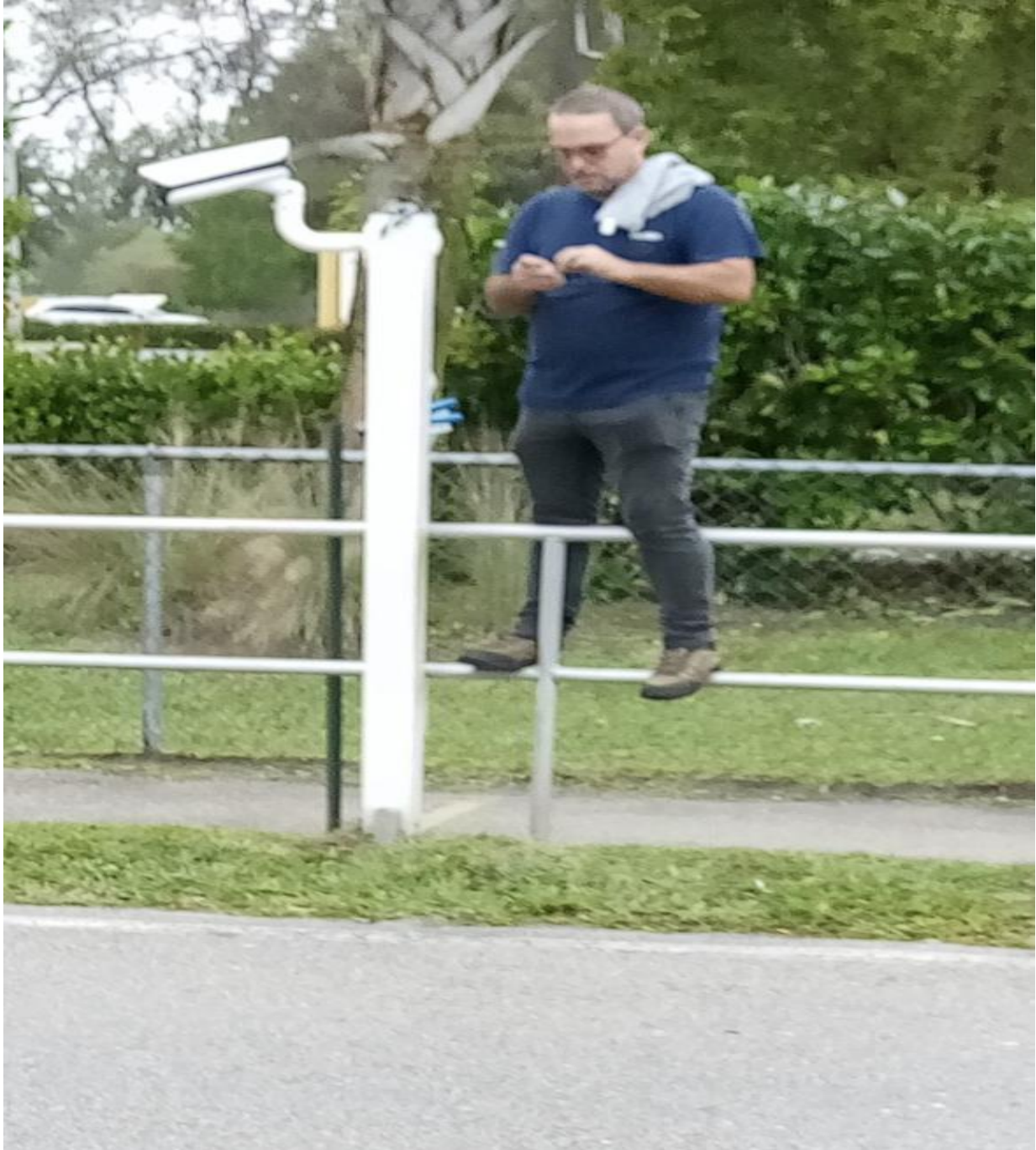
OKEECHOBEE BOULEVARD ENTRANCE- NEW CAMERAS WERE INSTALLED BY ACCESS MASTERS ON 1/23.
