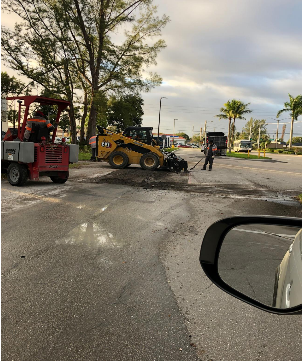
WEST DRIVE- LAST WEEK, ATLANTIC SOUTHERN PAVING MADE REPAIRS TO ROADS AT VARIOUS SECTIONS OF CV.
