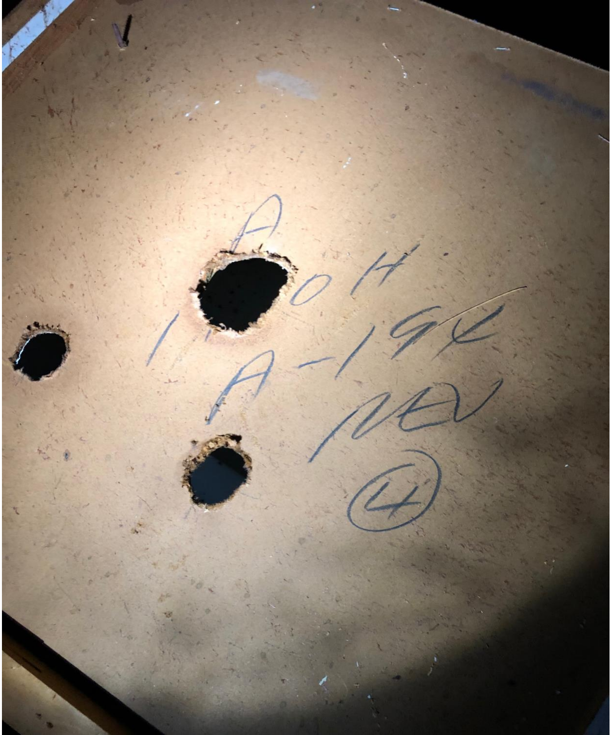
ANDOVER H- ORIGINAL CV CABINETS ARE MARKED WITH THE UNIT NUMBER. IN THIS CASE, 194 ANDOVER H.
