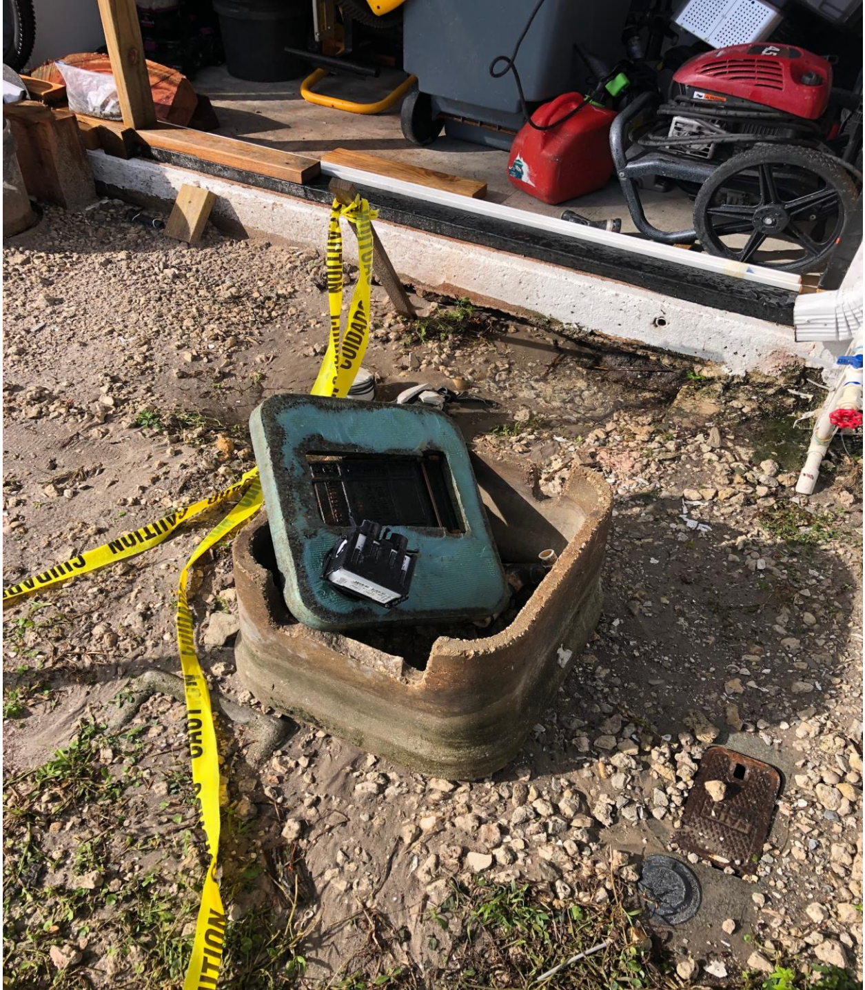
128 NORTHAMPTON G- FOR SOME REASON, THIS WATER METER BOX WAS REMOVED, AND THE USAGE METERS FOR TWO UNITS WERE DISCONNECTED. PBC WATER HAS BEEN NOTIFIED.
