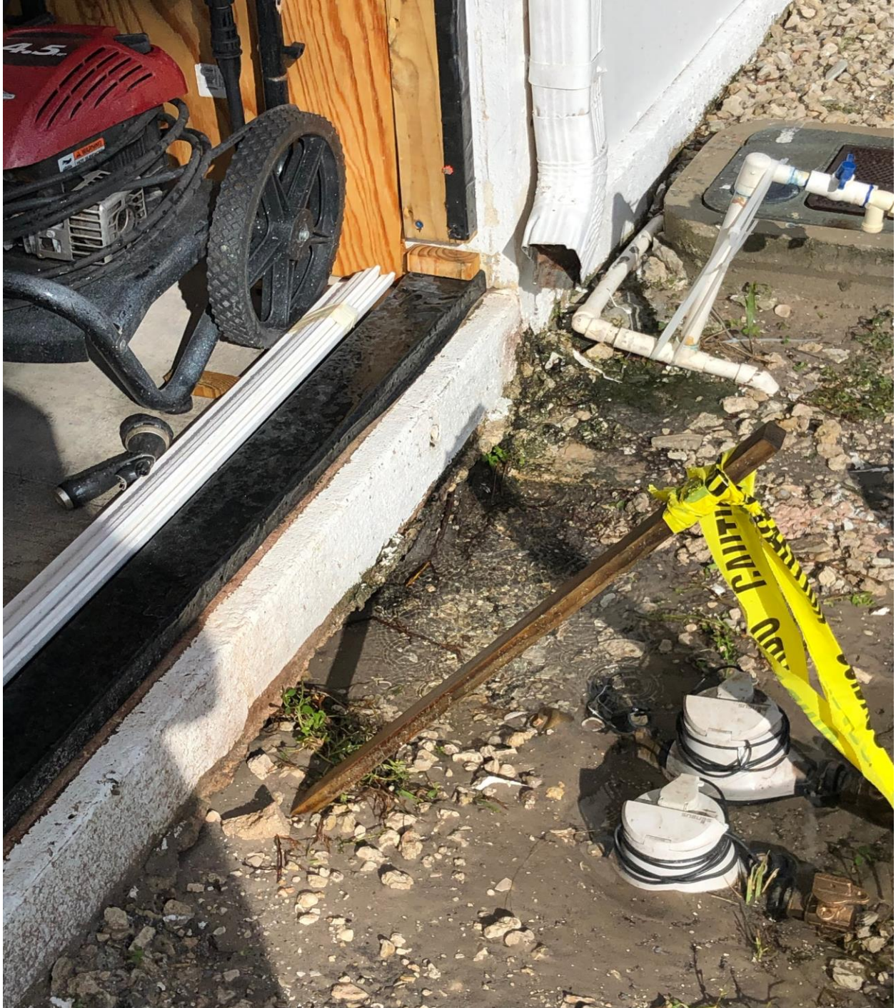
128 NORTHAMPTON G- WATER FROM A ROOF GUTTER DOWNSPOUT IS UNDERMINING THE FOUNDATION OF THIS BUILDING.
